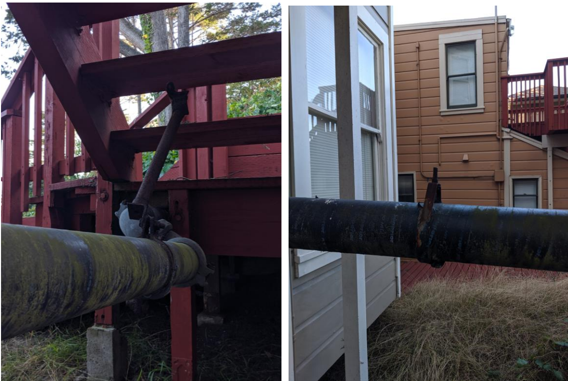
Figure 10 - Unattached, Corroded Water Pipe Brace and Hanger
