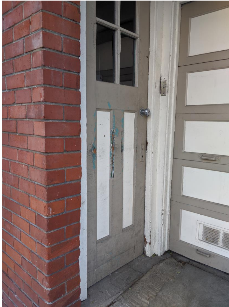
Figure 5 - Wood Deterioration at Garage Door
