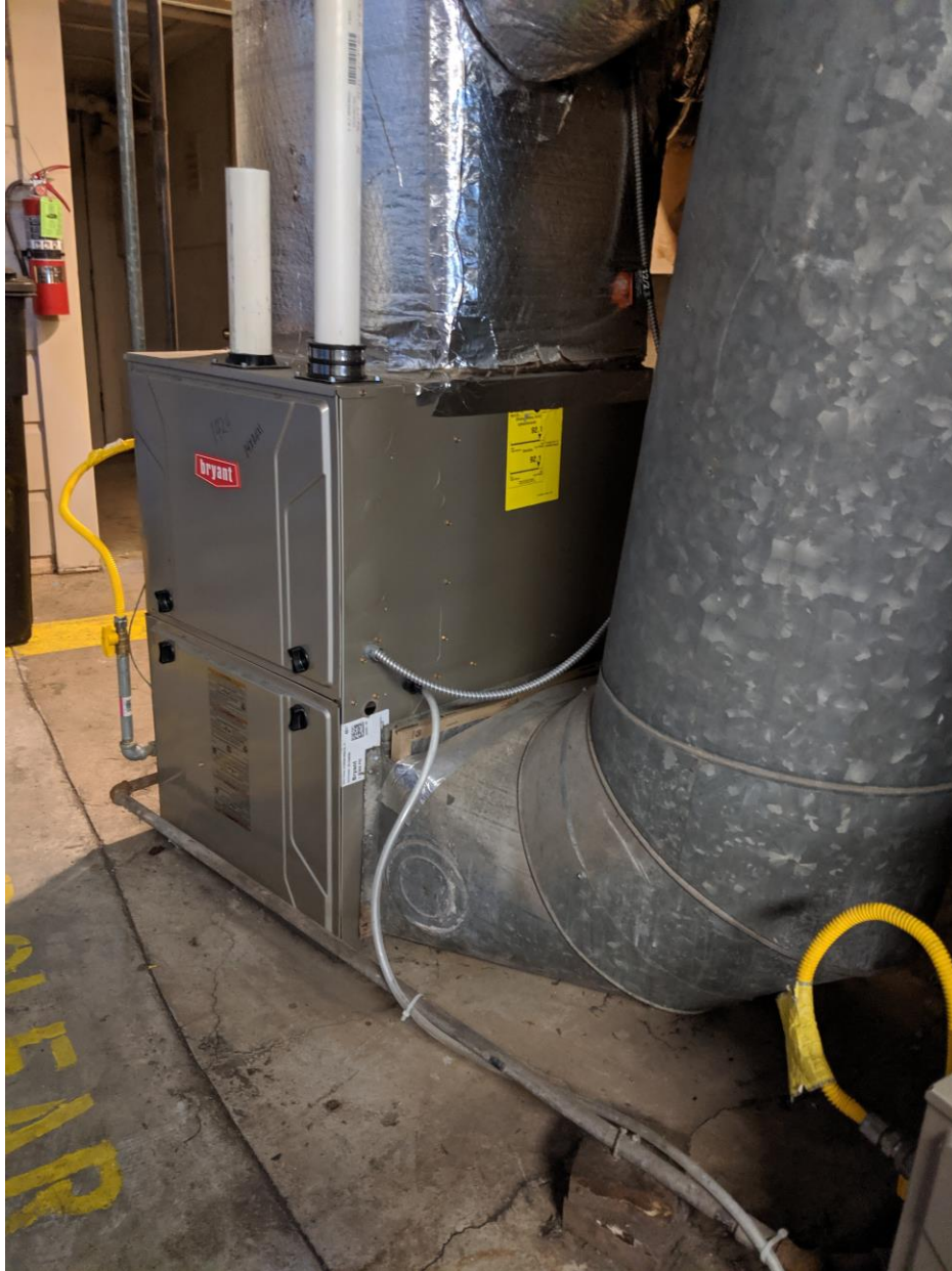
Figure 8 - Gas Furnace in Garage
