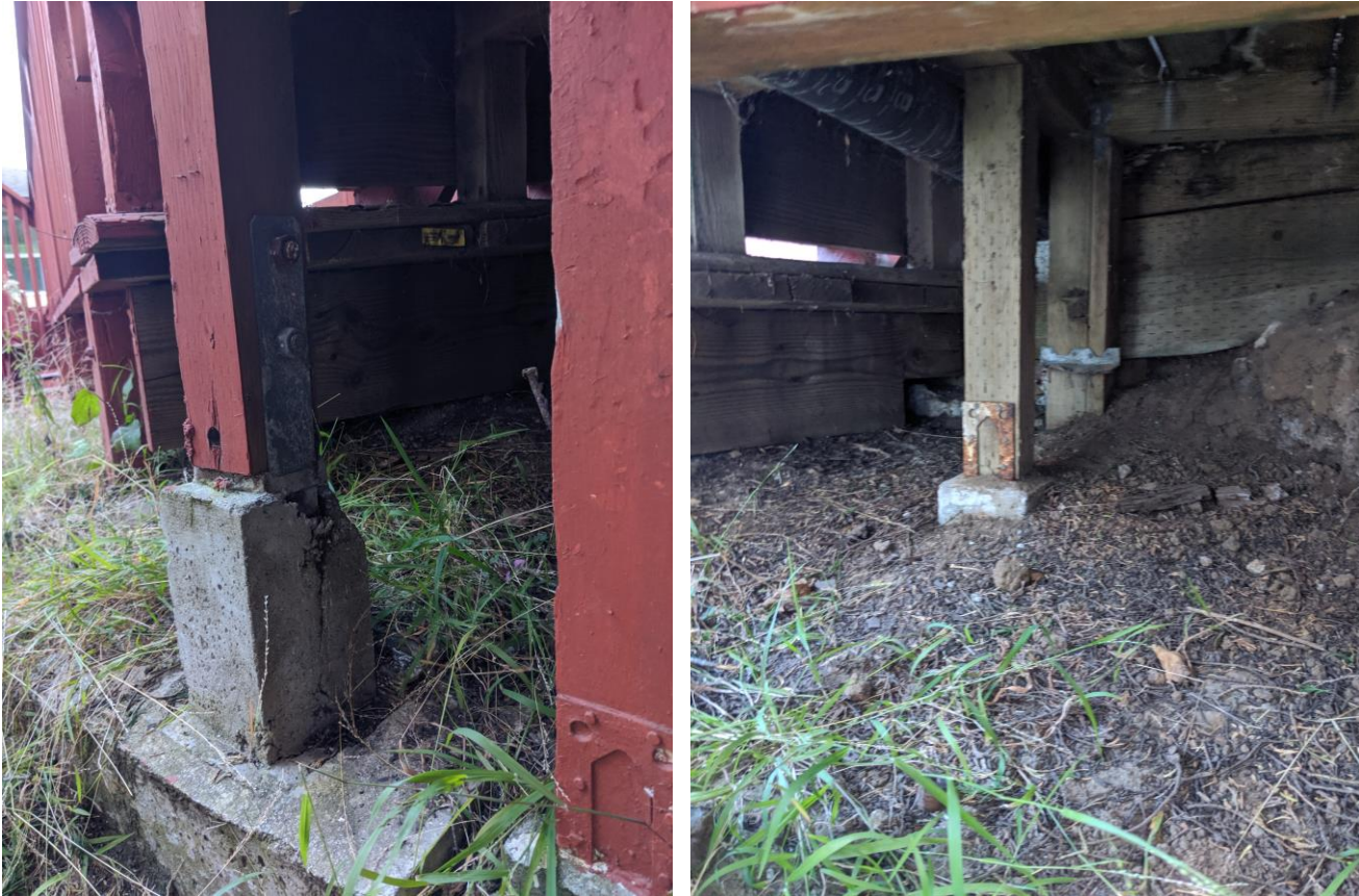
Figure 11 - Corrosion Observed at Elevated Wood Walkway
