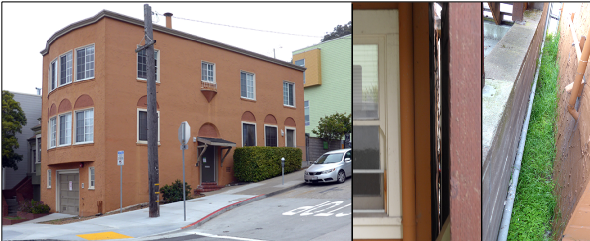
Center image is separation gap from building on the north and left image is the separation from retaining wall to the east.
