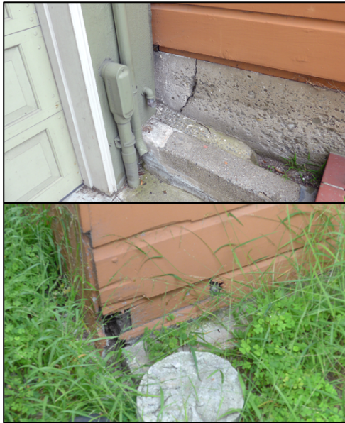
Figure 3. The upper image shows the bottom section of the north party line wall foundation and original straight-board sheathing. The lower image is of the corner of the building to the right of the above image.
