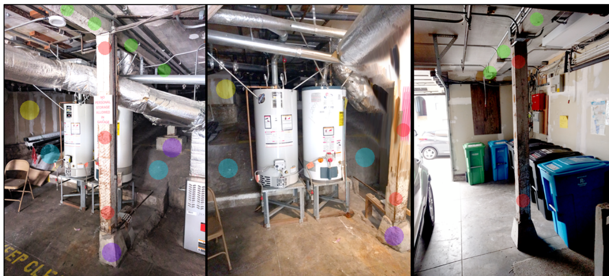
Figure 2. Interior images of the first story showing the framing of the interior, and the water heaters. The left and right images are in opposite longitudinal directions. The green dots indicate dimensional lumber beams, the red are dimensional lumber posts, the purple are the footings, the blue is a low transverse stem wall, and the yellow is gypsum board installed at some locations when the fire sprinklers were installed. In the middle image note the diagonal braces from the ceiling to the water heaters.
