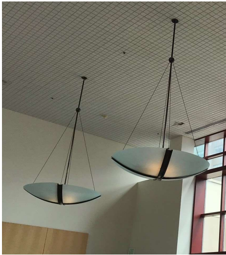
Lighting, 5 th floor lounge area
