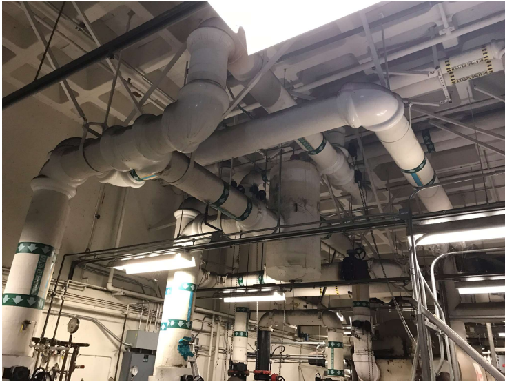
Absorption chiller piping at level E (1 st floor slab above)
