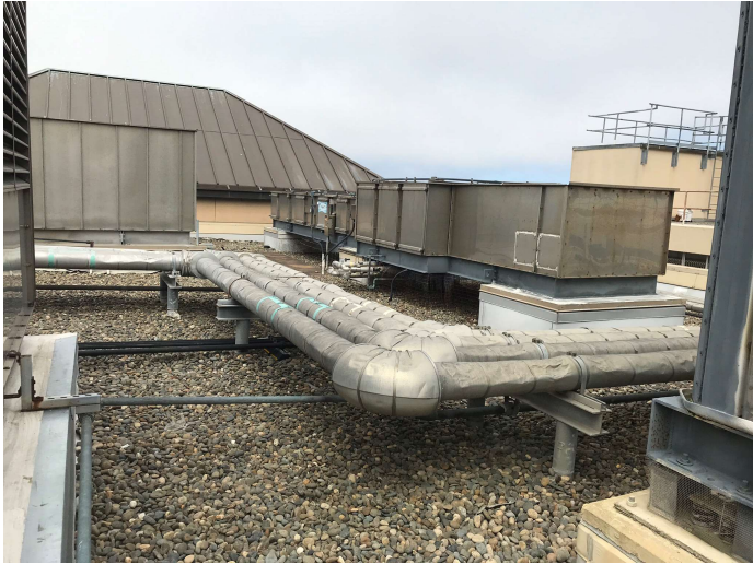
Roof membrane ballast, AHUs, and piping
