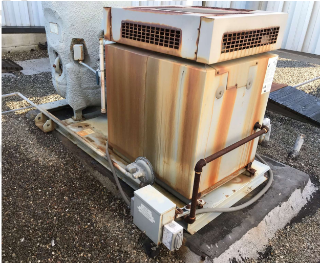
Rooftop boiler for domestic hot water
