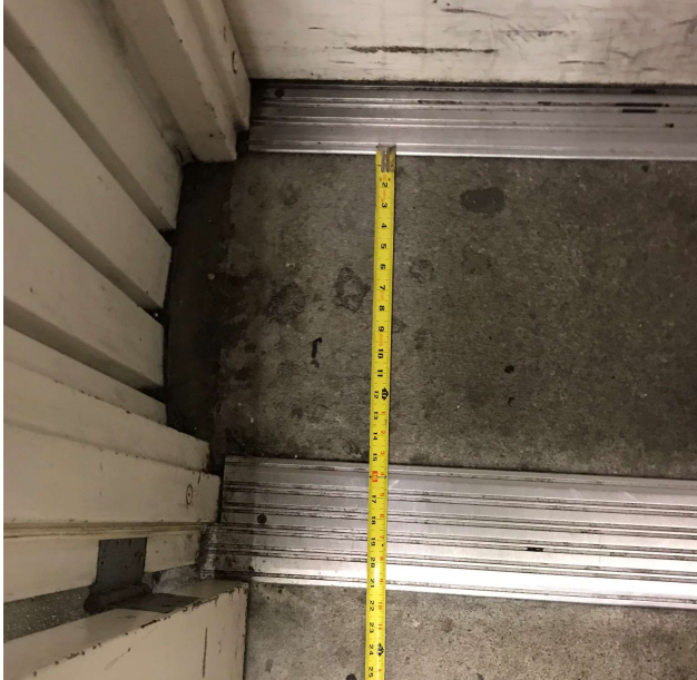
Threshold at entrance from parking garage (seismic separation joint cover at left)
