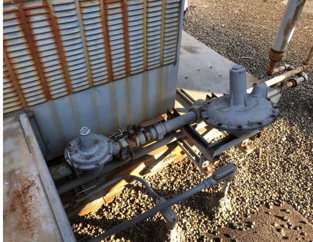
Natural gas line to HVAC boiler
