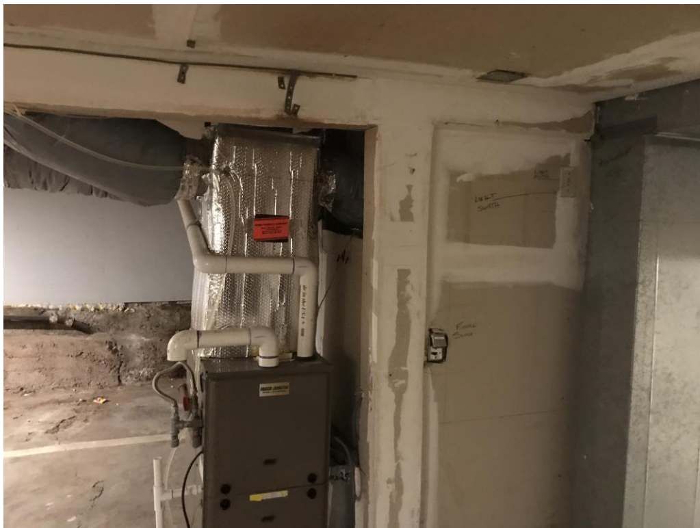
Figure 9 – Furnace in Basement
