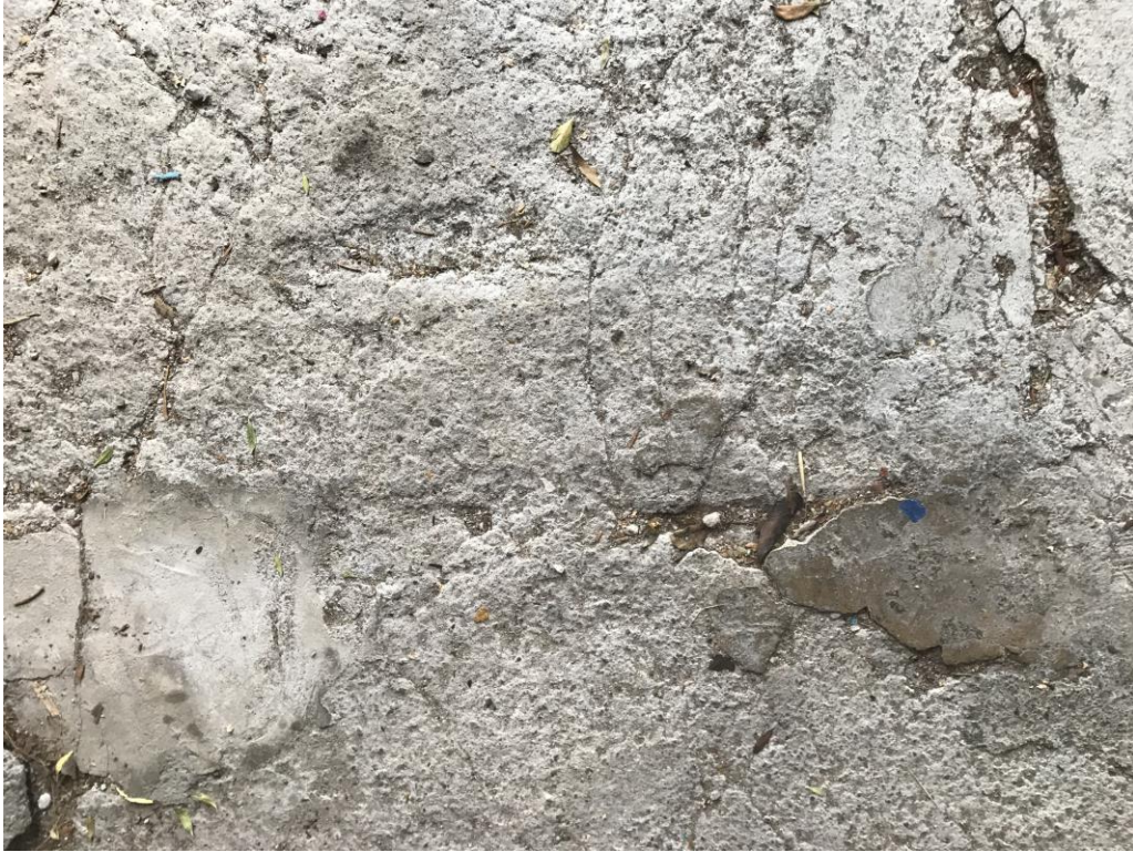
Figure 6 – Concrete Spalling of Garage Slab
