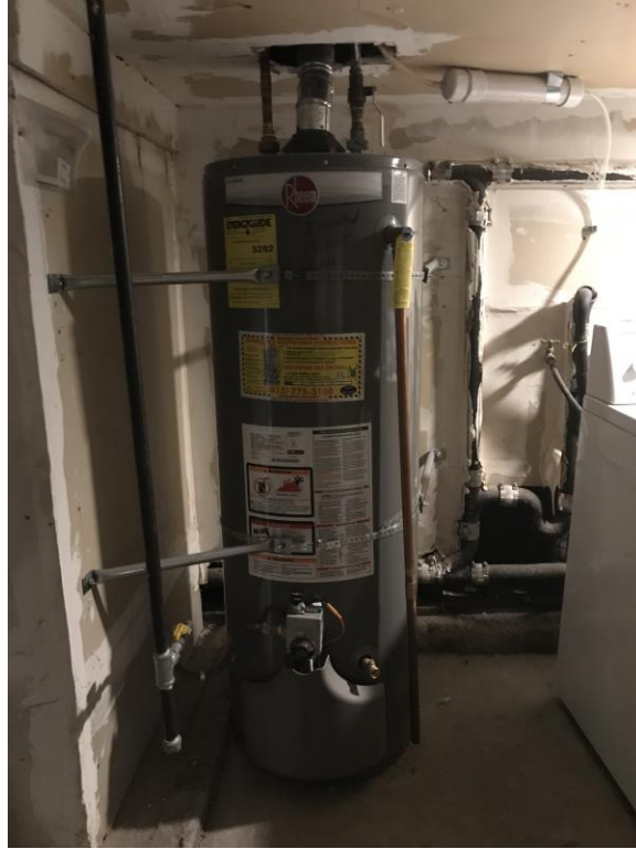
Figure 8 – Anchored Water Heater
