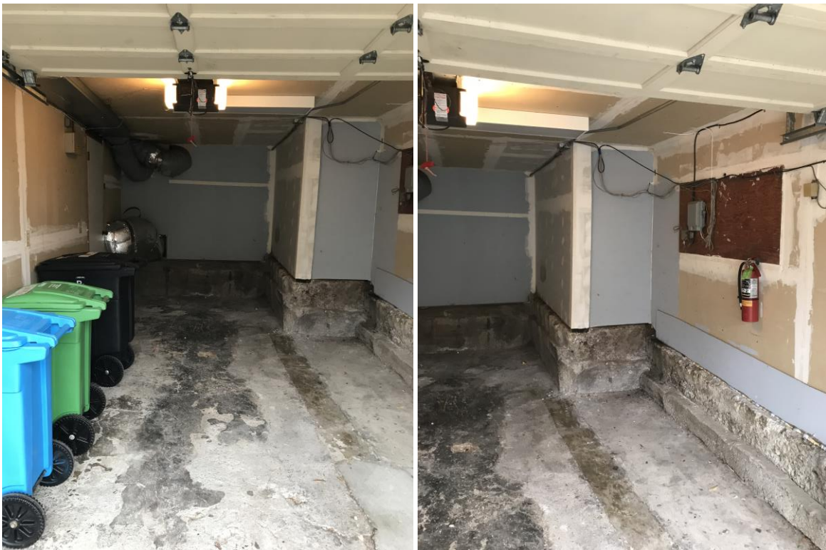
Figure 5 – Concrete Spalling at Garage
