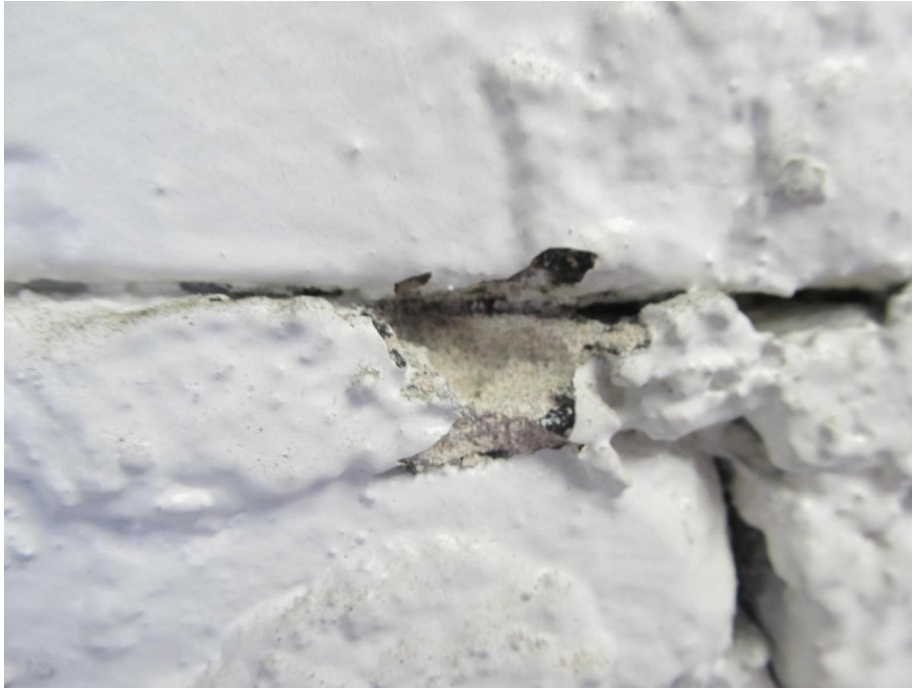
Scraped mortar of URM wall using flat-head screwdriver on southeast corner of building at the first story
