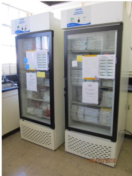
Unbraced refrigerators in laboratory with biohazard tag at second story (looking northeast)
