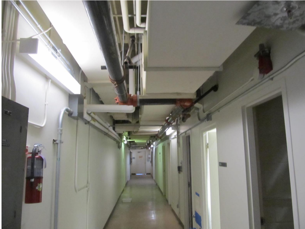
Corridor at second story with hollow clay tile partitions on the right side (looking east)
