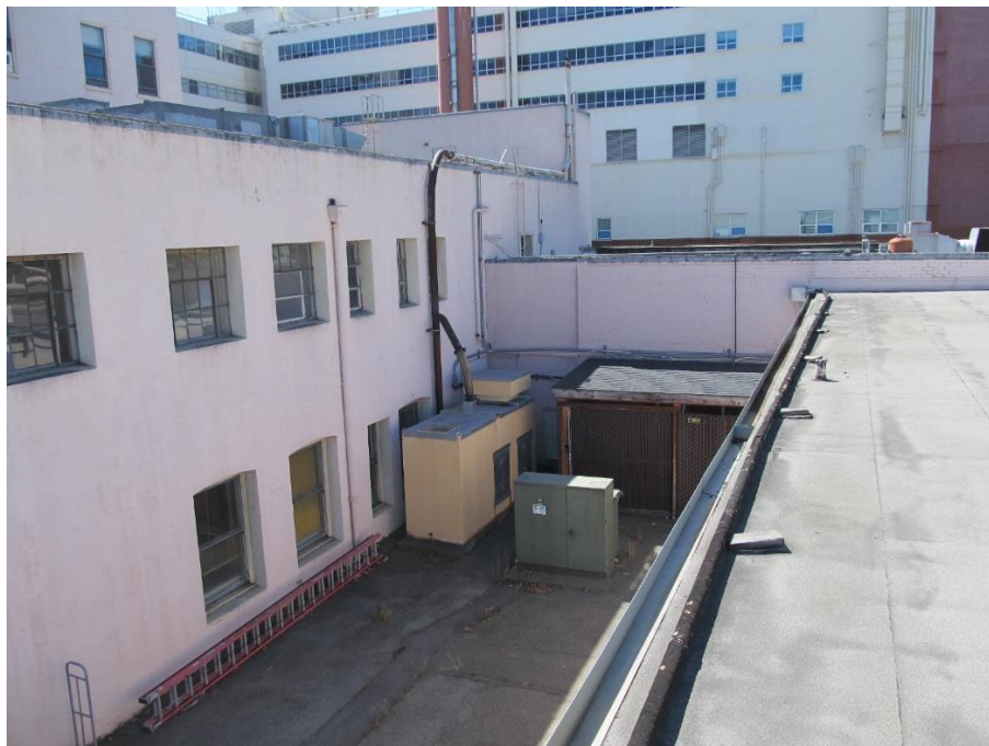
Re-entrant corner at north elevation of the south wing and east elevation of the north wing (looking southwest from Building G)
