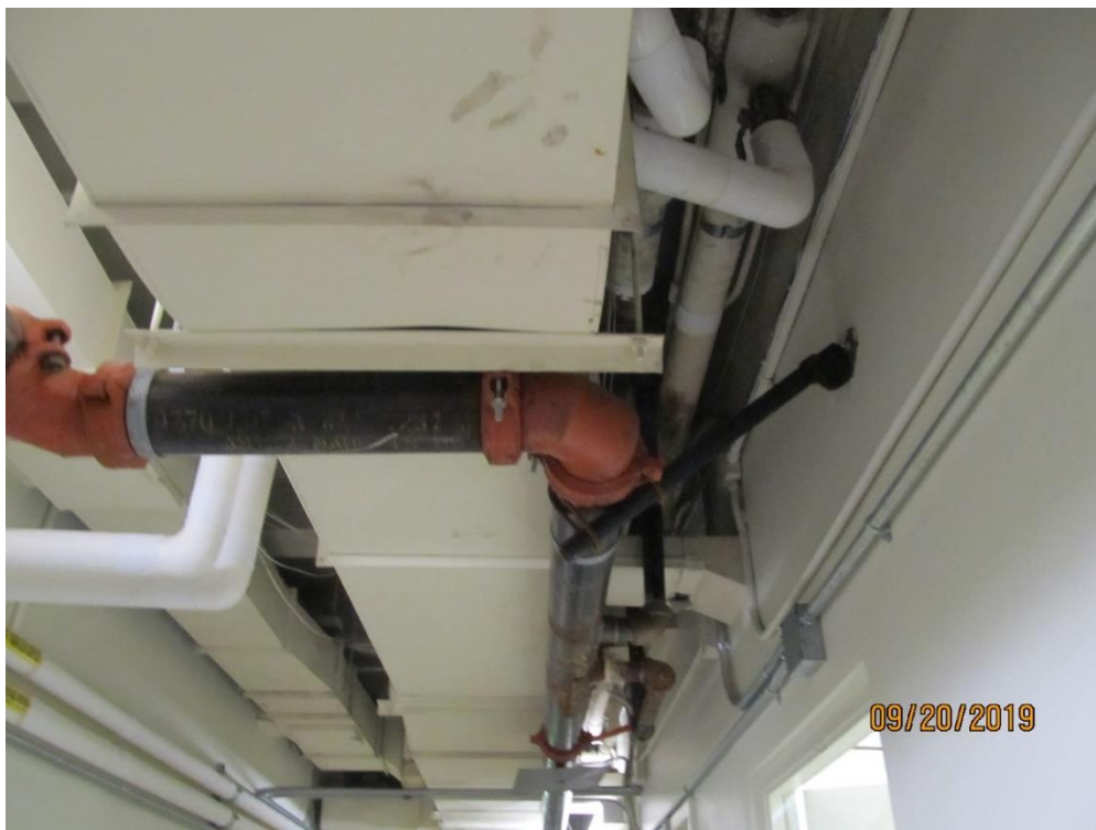
Pipe system braced to the hollow clay tile partitions at second story
