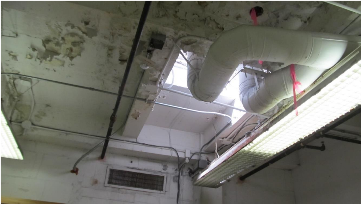
Water damage due to deficient waterproofing on south wing
