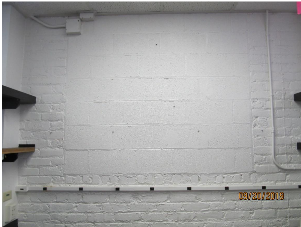
Original URM masonry walls with CMU infill after the 1962 alterations at second story
