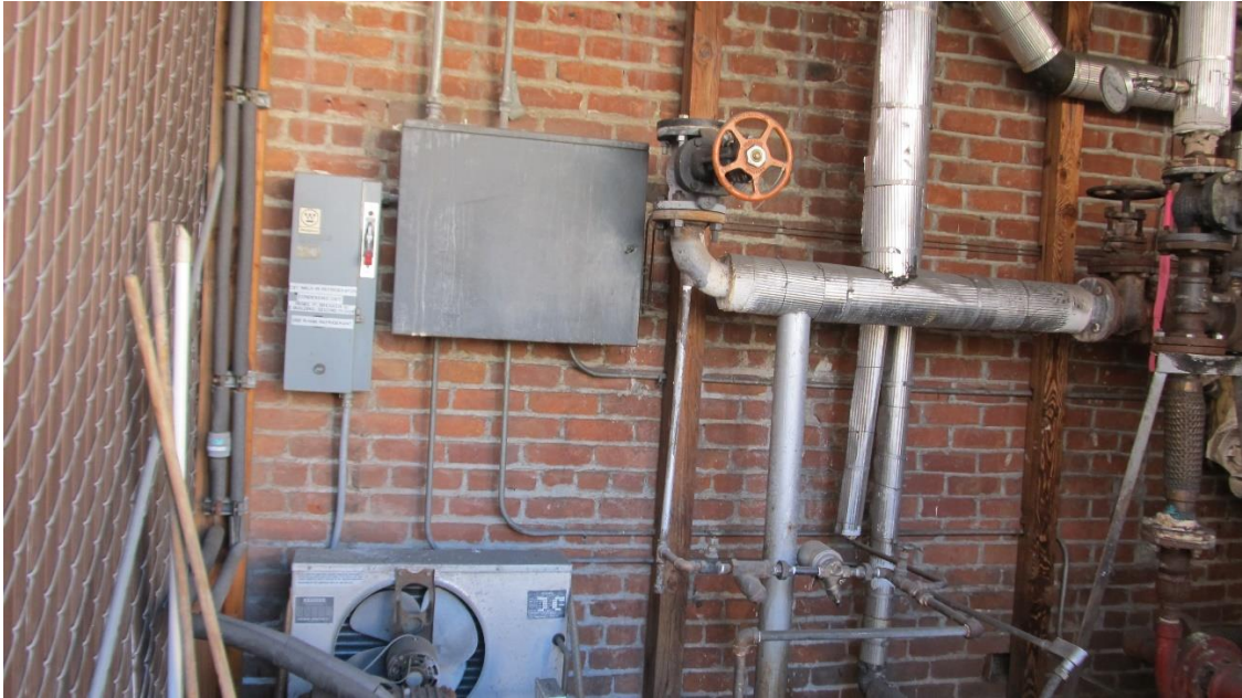
Exposed solid clay URM wall at east elevation of north wing (looking west)
