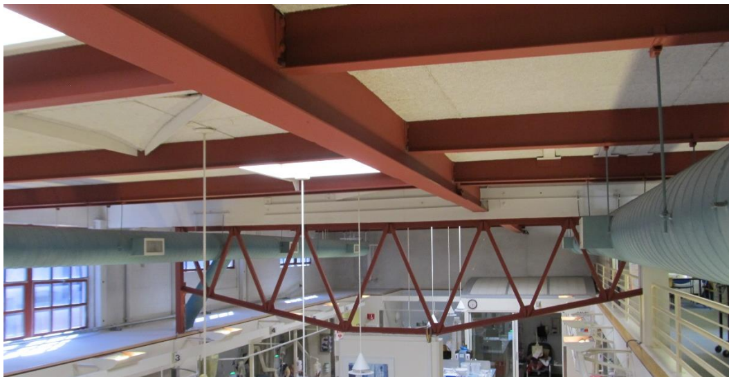
Looking southwest at interior truss at shear wall. The soffit attached to the south wall that is located over patients is on the left and the mezzanine slab attached to the north wall is on the right.
