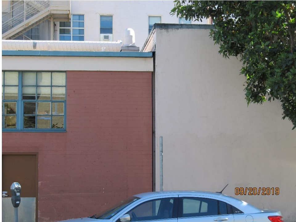
Seismic joint between Building G and Building E looking south (Building G on the left and Building E on the right)
