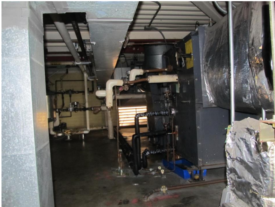
Mechanical room on the second-floor east mezzanine (looking south)
