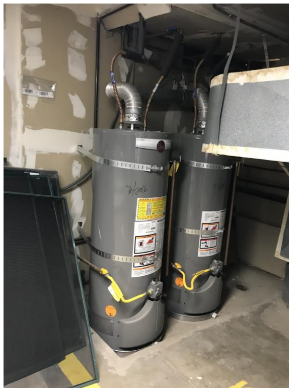
Figure 11 – Braced Water Heaters
