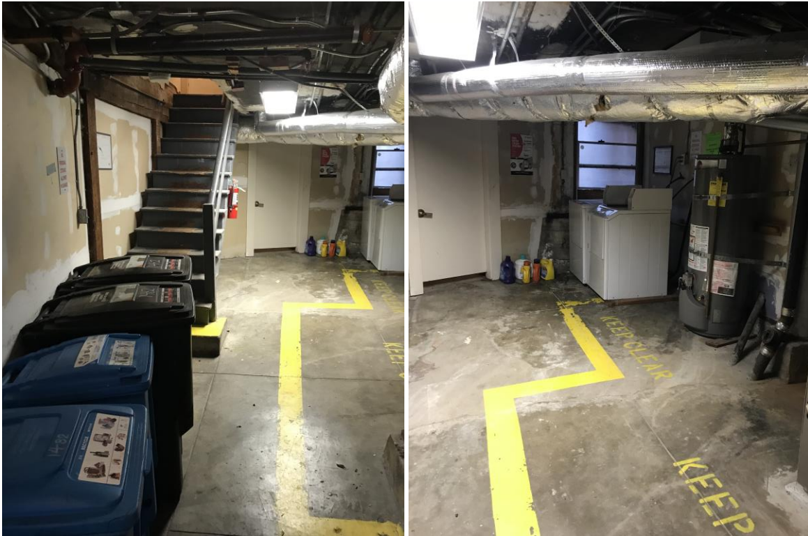
Figure 9 – Furnace / Laundry Room
