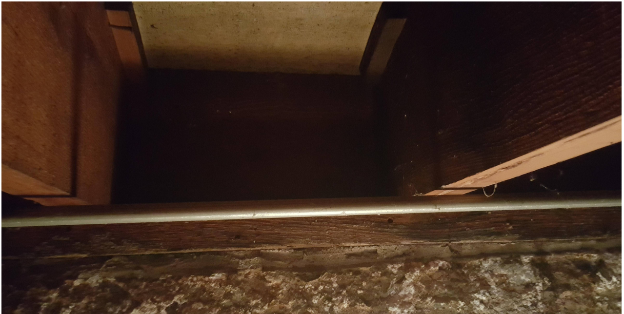
PHOTO - 1st Floor Framing (2x12@16" O.C.) on Sill Plate with not Shear Connection to Foundation
