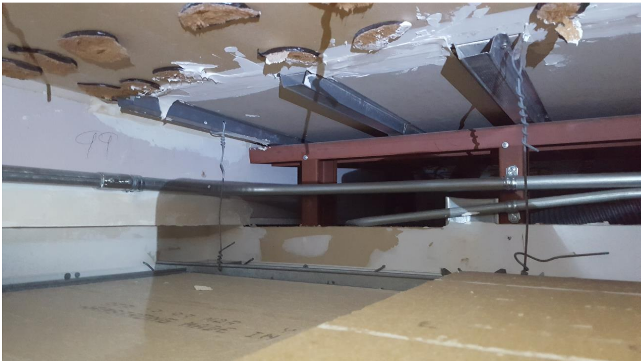
Figure 7 - Interior Partition Wall with Gypsum Board Sheathing Stopping Below Structure
