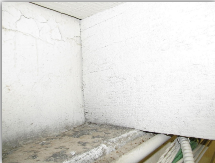
Photo A1: Wood joist bearing on south concrete wall ledge with no positive connection (inside face of concrete parapet to the left and wood joist to the right)
