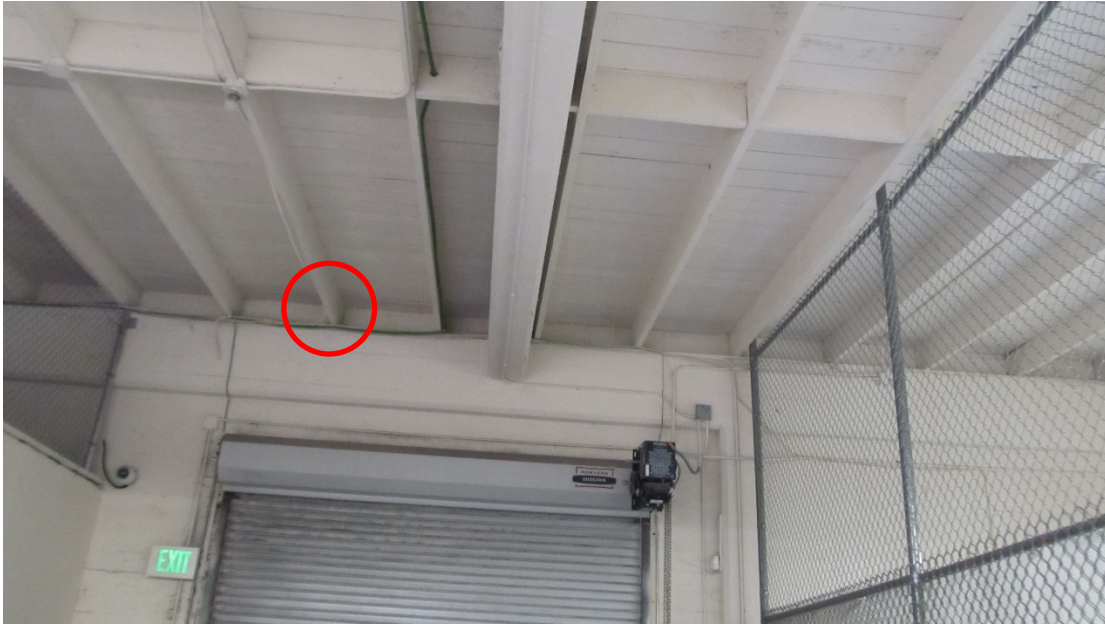
Photo A: Wood joist bearing on south concrete wall ledge with no positive connection (see close-up of circled connection in Photo A1 below)
