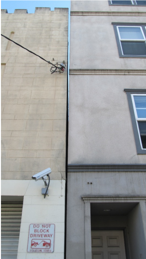
Separation gap on north elevation (looking south)
