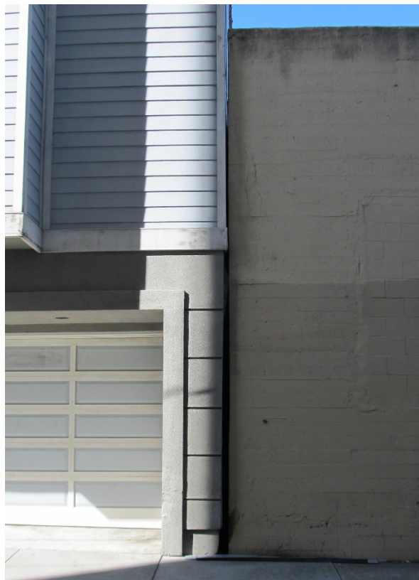
Separation gap on south elevation (looking north)
