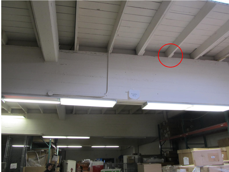
Photo B: Interior wood joist bearing on concrete girder with no positive connection (see close-up of circled similar connection in Photo B1 below)
