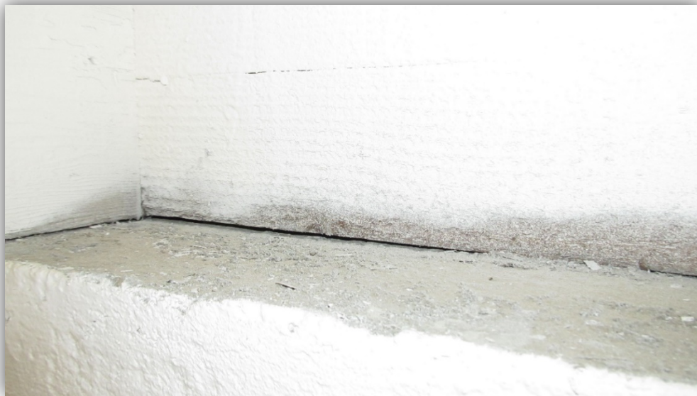
Photo B1: Interior wood joist bearing on concrete girder with no positive connection (wood blocking to the left and wood joist to the right)
