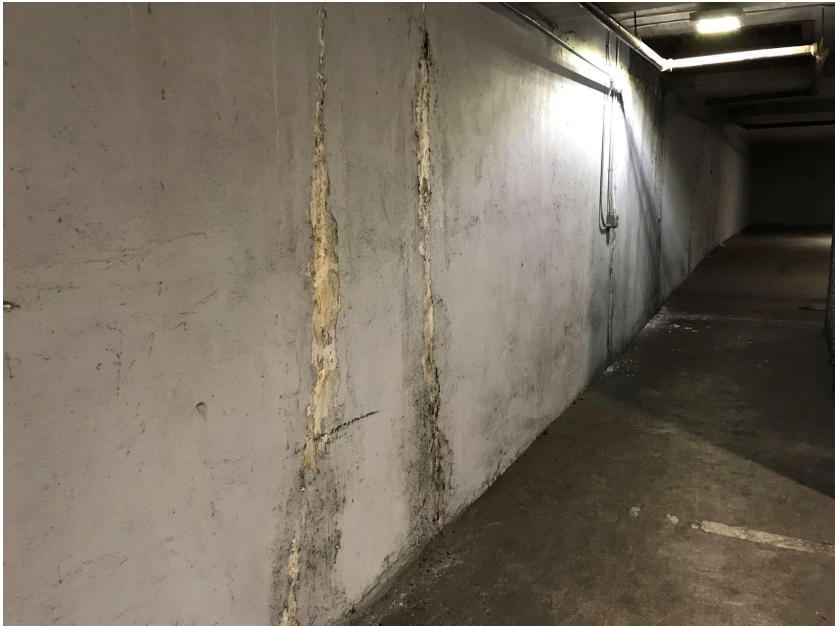
Level B4 perimeter wall with evidence of moisture intrusion
