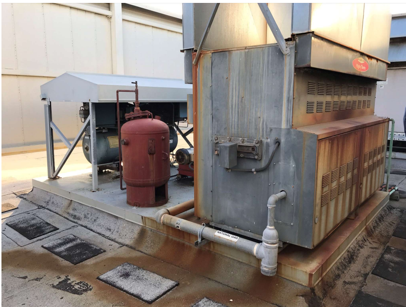
Gas-fired HVAC boiler – high roof
