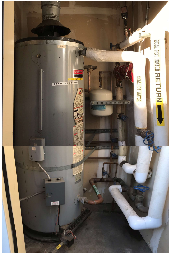
Gas-fired domestic water heater – high roof
