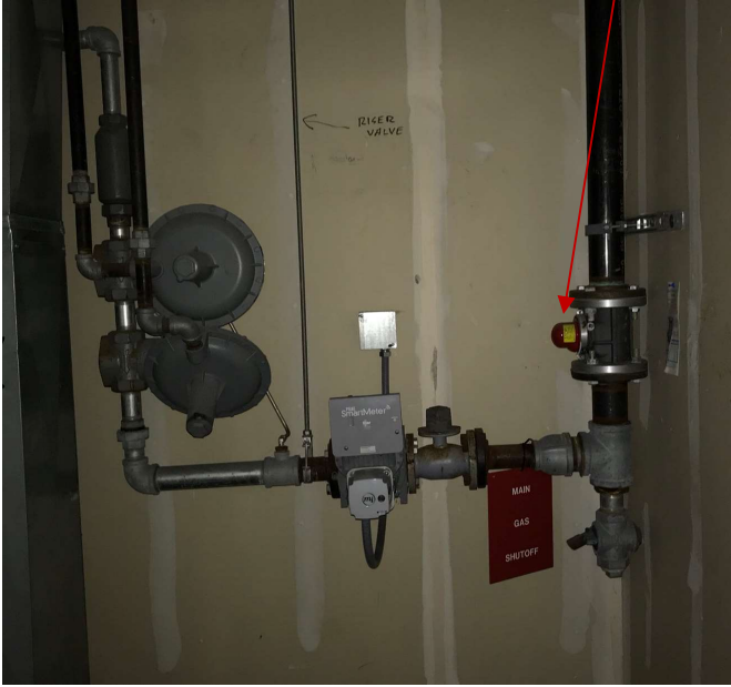
Gas main service shut off – Level B1
