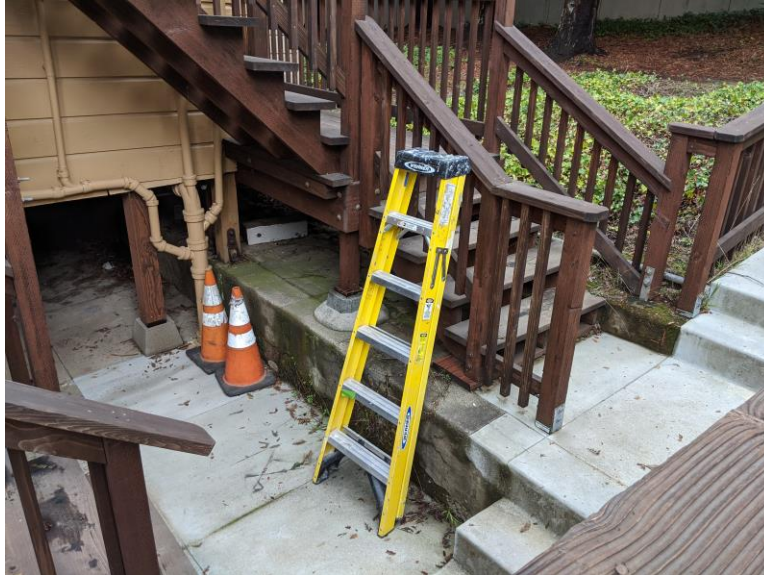
Figure 10 – Exterior Wood Stairs and Elevated Rear Addition on Posts
