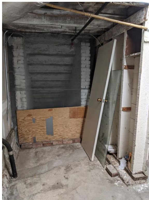
Figure 7 – Underside of First Floor Entrance Stairs and Backside of Interior Partition
