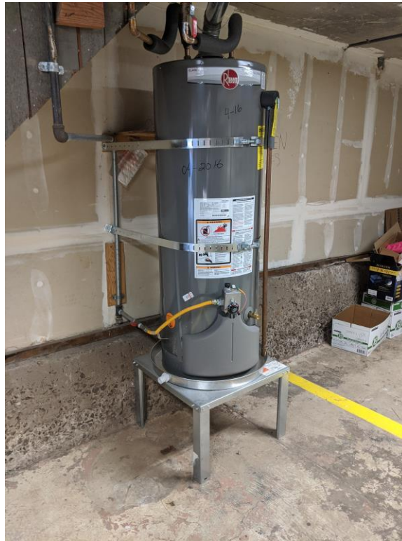
Figure 8 – Anchored Water Heater, Concrete Stem Wall, & Gyp Wall Sheathing
