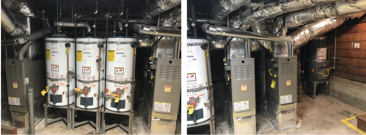
Figure 8 – Water Heaters and Furnaces in Utility Area
