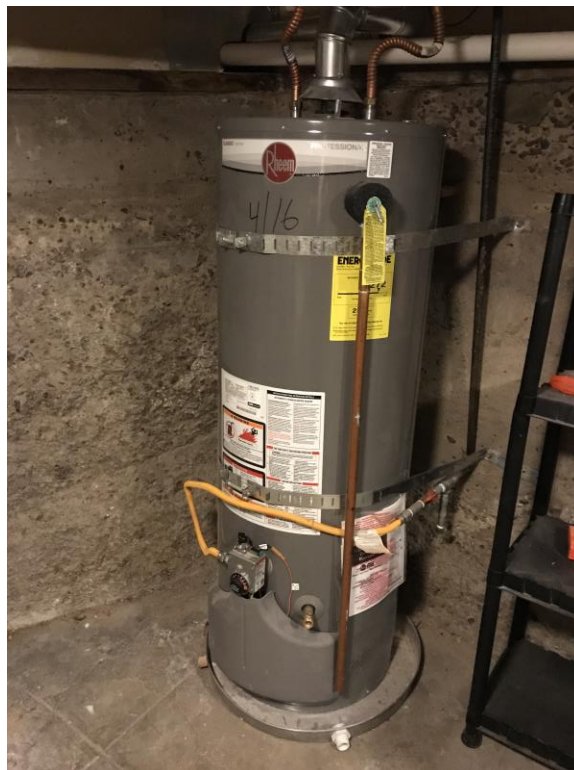
Figure 11 – Anchored Water Heater
