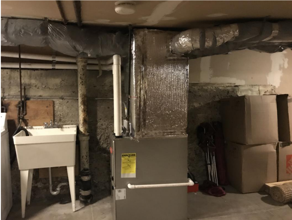
Figure 12 – Furnace in Basement
