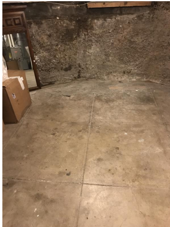
Figure 13 – Buckling in Basement Slab on Grade
