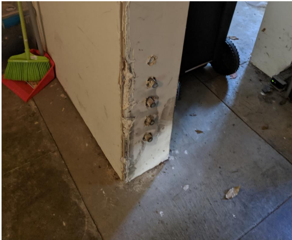
Figure 9 - Hold-down Bolts to Vertical stud and Extent of Foundation Element below Wall on Gridline 1
