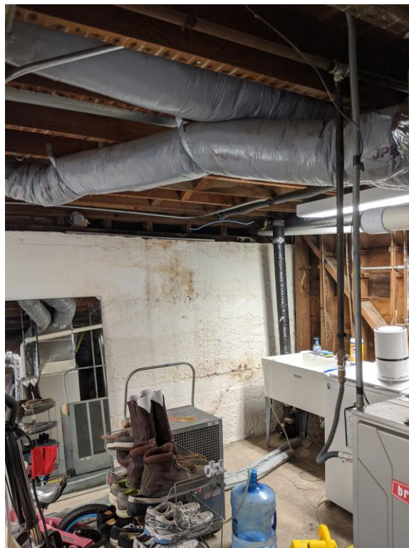
Figure 7 – East Rear Wall (Left) and Let-In Wall Bracing on South Wall (Right)
