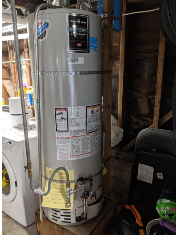
Figure 8 – Anchored Water Heater
