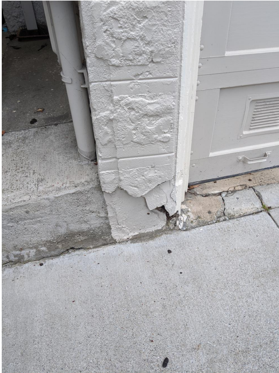
Figure 5 – Damage to Northwest Corner Veneer
