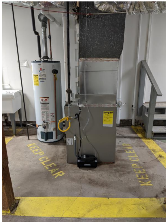
Figure 14 – Unrestrained Water Heater and Furnace at Basement
