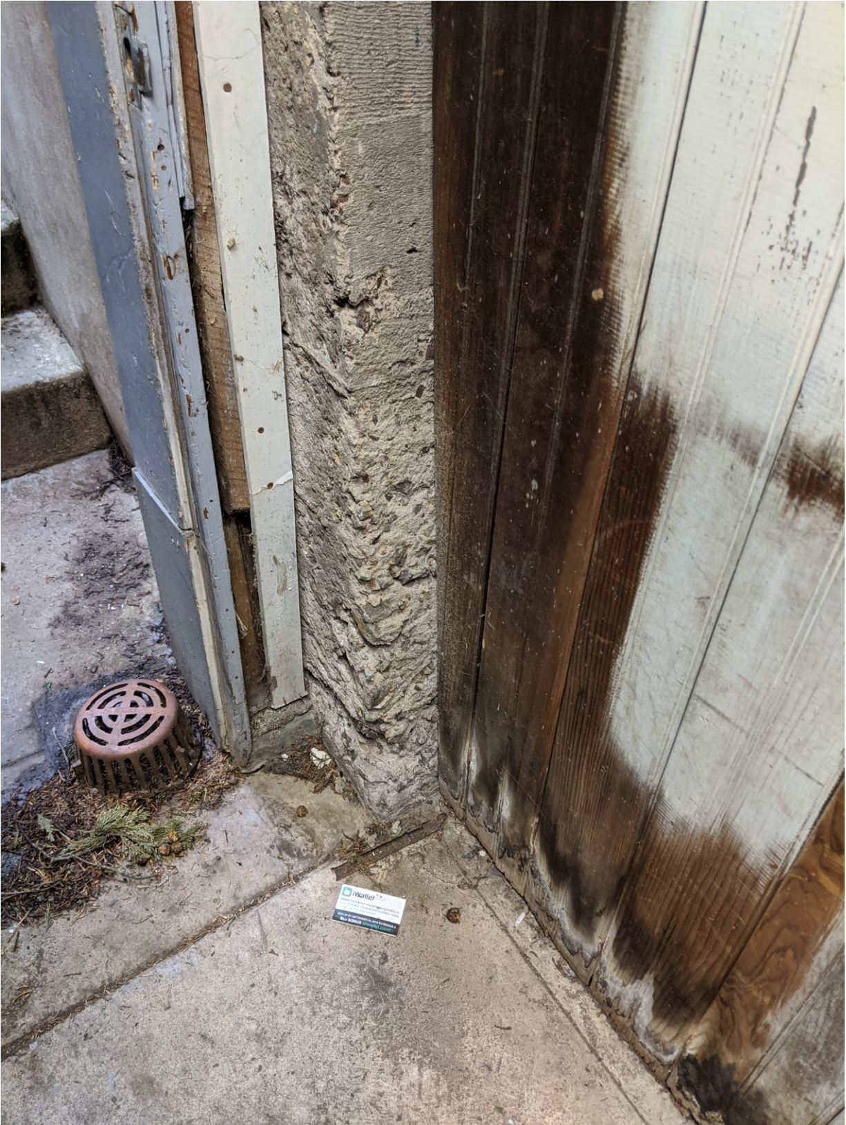
Figure 10 – Condition of East Basement Stem Wall
