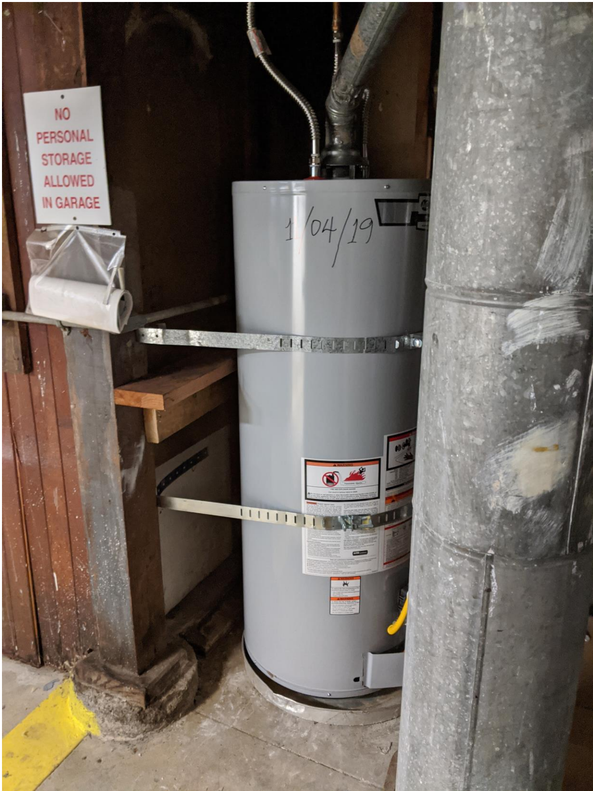
Figure 8 – Braced Water Heater in Basement
