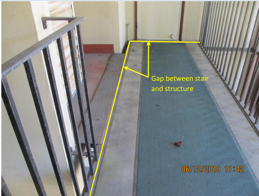
Stair between original 1954 structure and the 1964 lab addition (looking west at the east elevation of the original structure)
