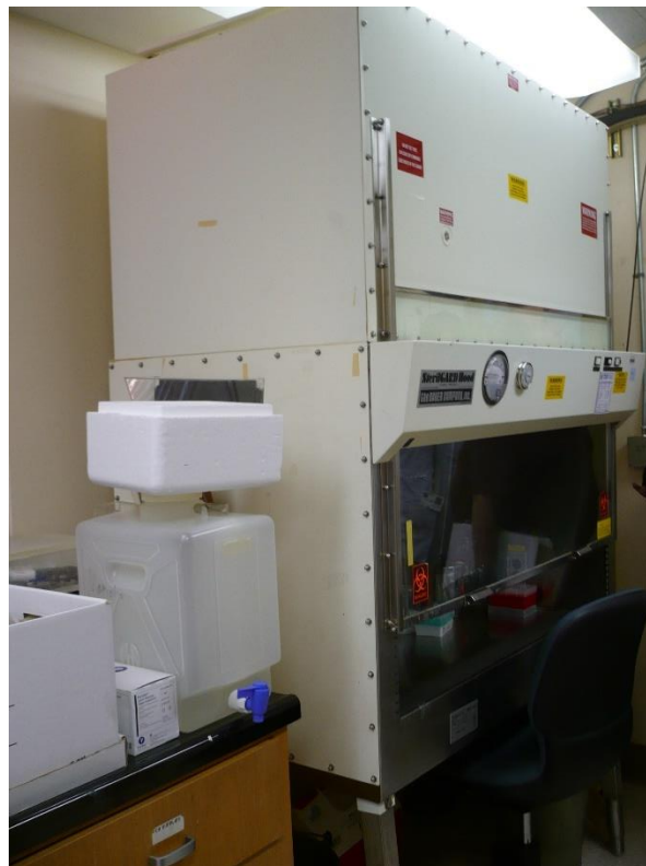
Unbraced fume hood
