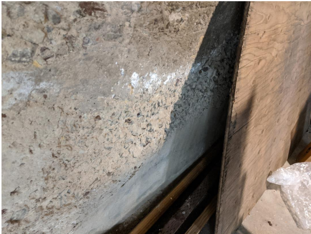
Figure 9 - Concrete Stem Wall Spalling
