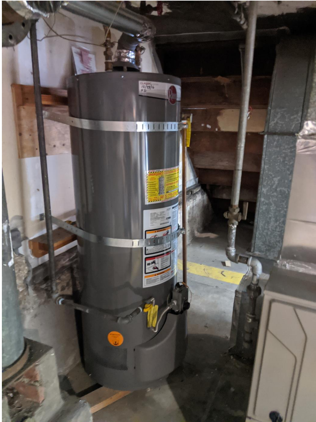
Figure 11 - Braced Water Heater in Basement
