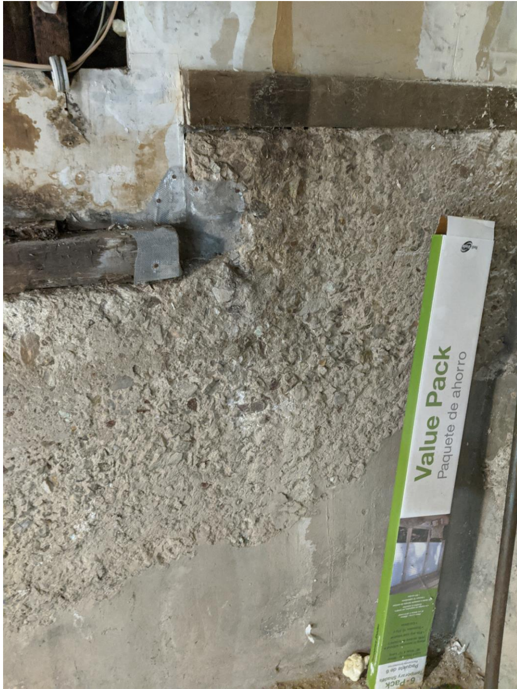
Figure 10 - Concrete Stem Wall Spalling
