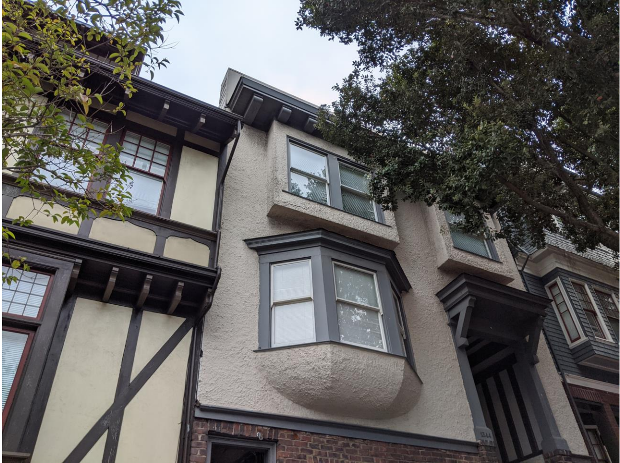
Figure 5 – Front Wall Condition
