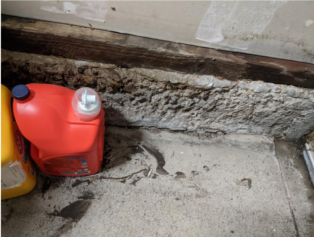
Figure 8 – Concrete Stem Wall Spalling
