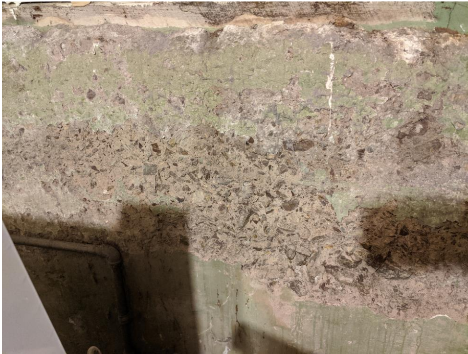
Figure 7 – Spalling of Concrete Stem Walls
