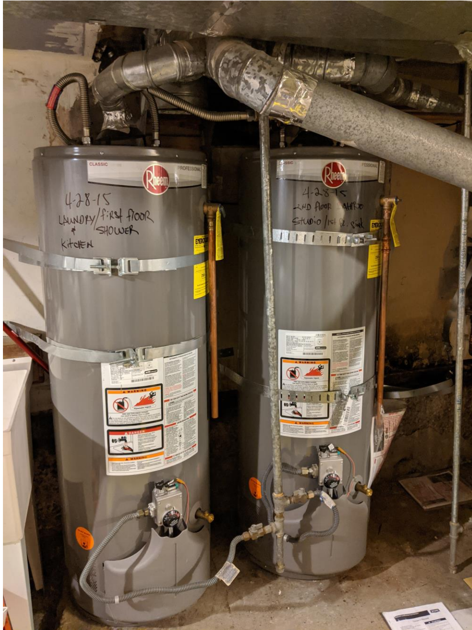
Figure 9 – Braced Water Heaters at Ground Floor Utility Space
