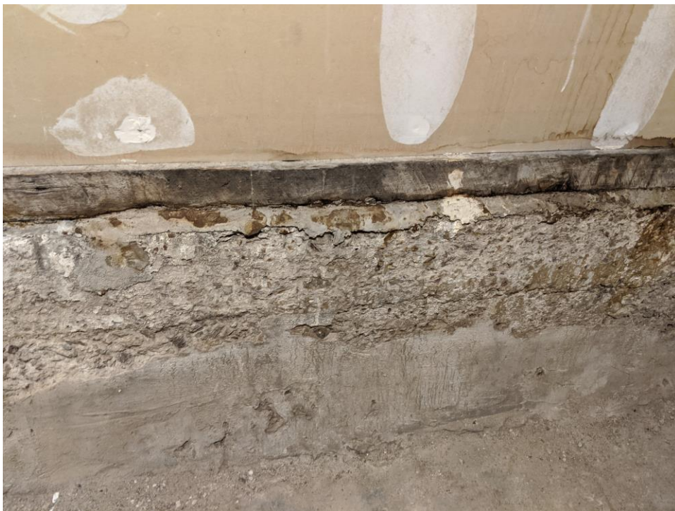
Figure 8 - Spalling of Concrete Stem Walls
