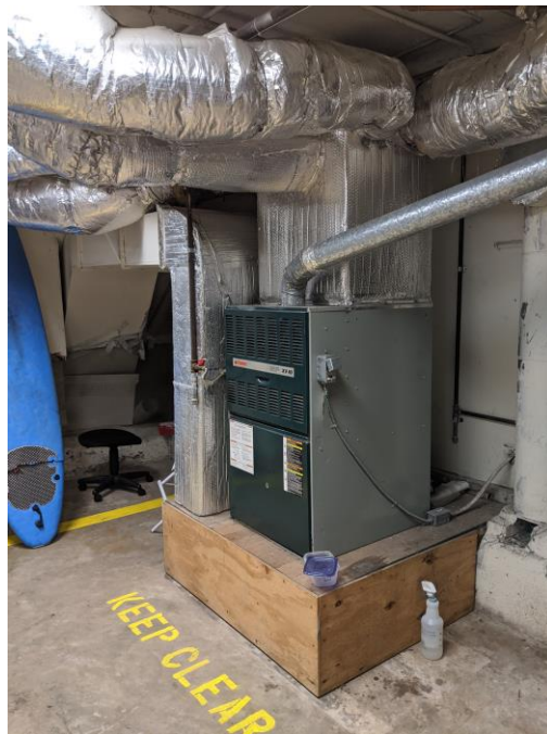
Figure 8 - Gas Furnace in Garage
