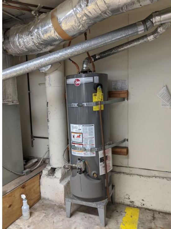
Figure 7 – Braced Water Heater in Basement
