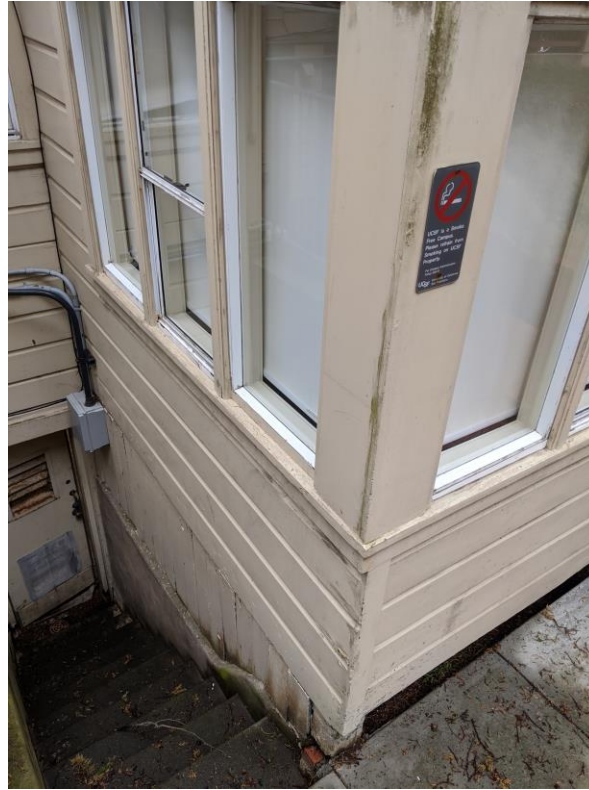
Figure 11 – Exterior Finish Condition at Rear of Building
