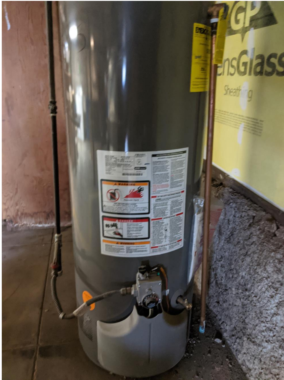
Figure 6 – Unanchored Water Heater in Basement
