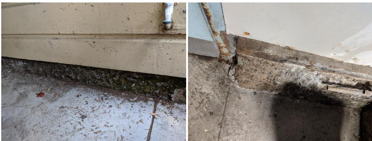
Figure 11 – Spalling of Concrete Stem Wall
