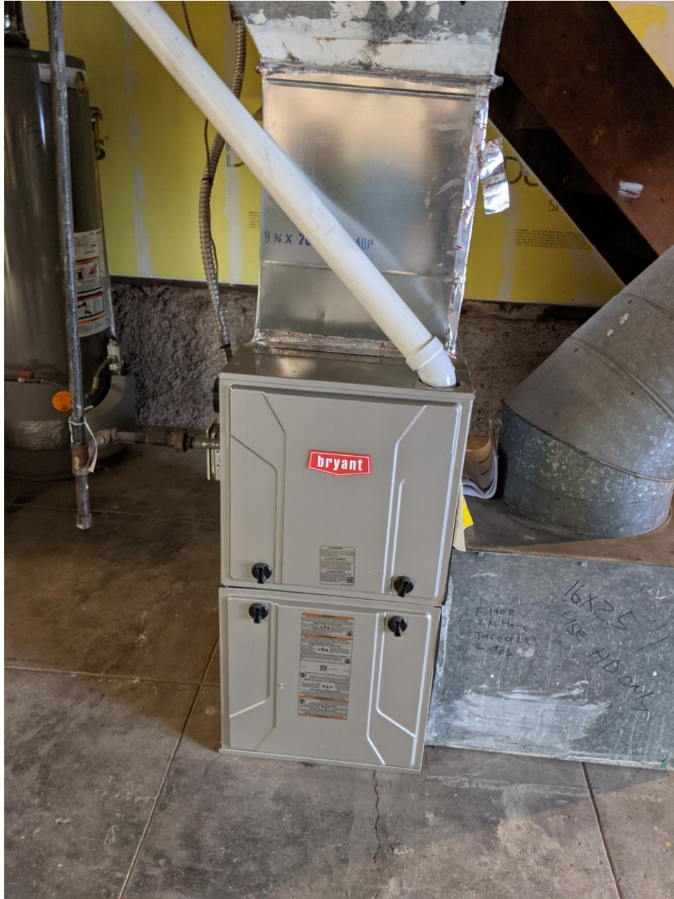
Figure 7 – Furnace in Basement
