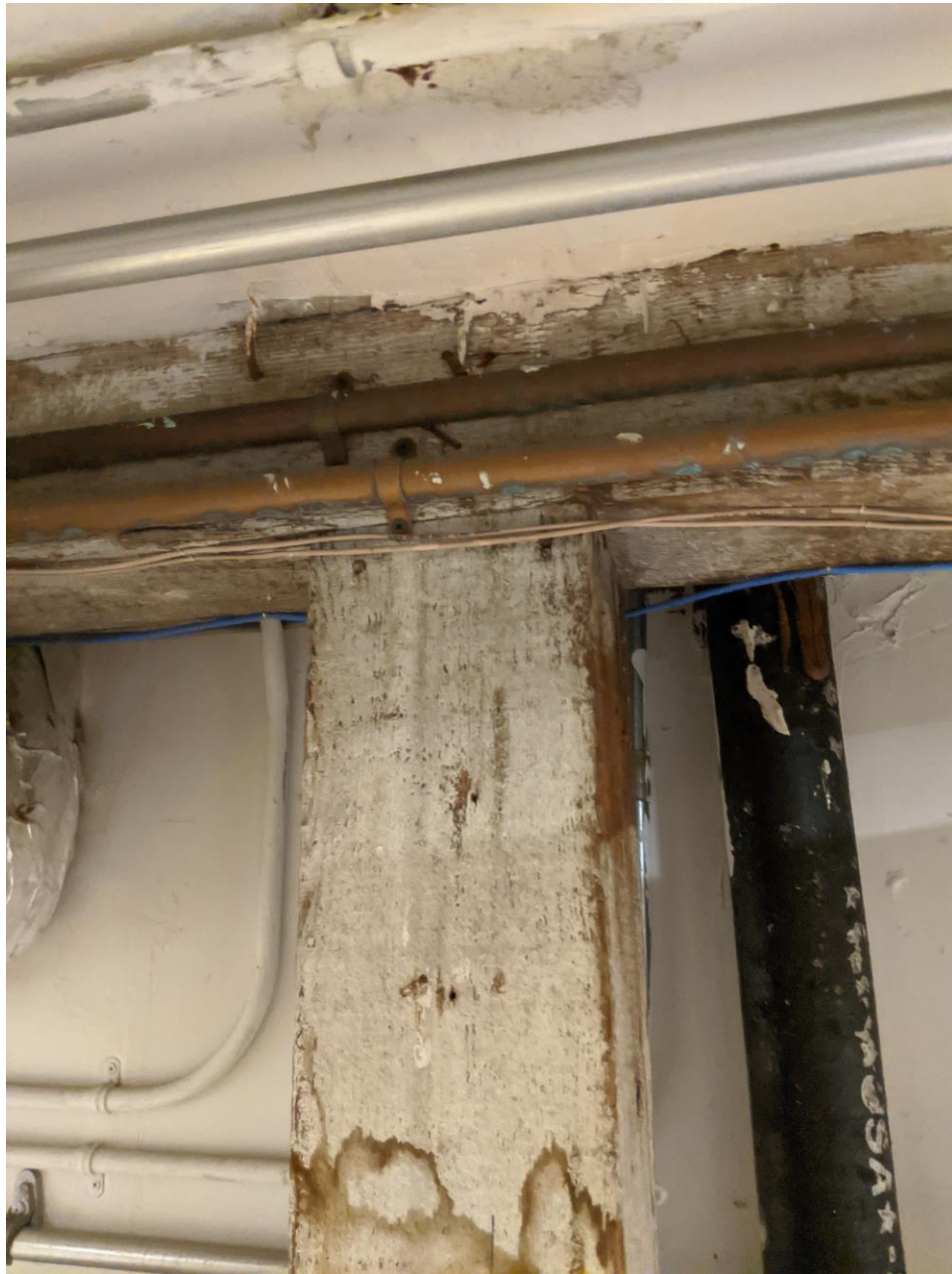
Figure 8 – Interior Basement Post and Beam without Positive Connections
