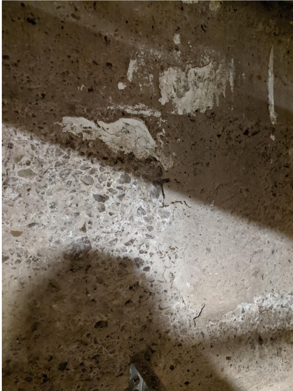
Figure 9 - Spalling of Concrete Stem Wall
