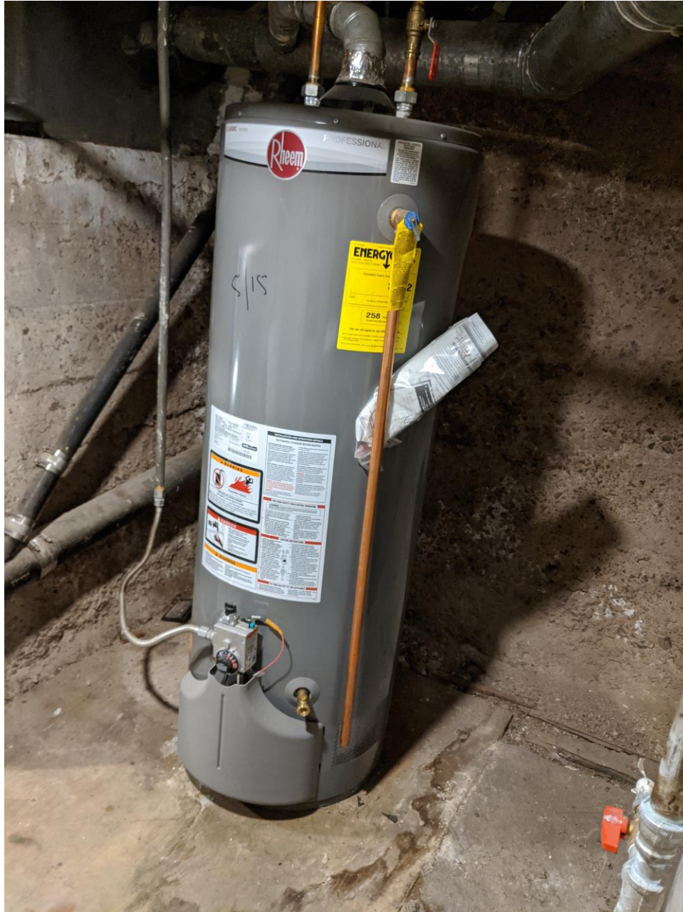
Figure 7 - Unanchored Water Heater in Basement
