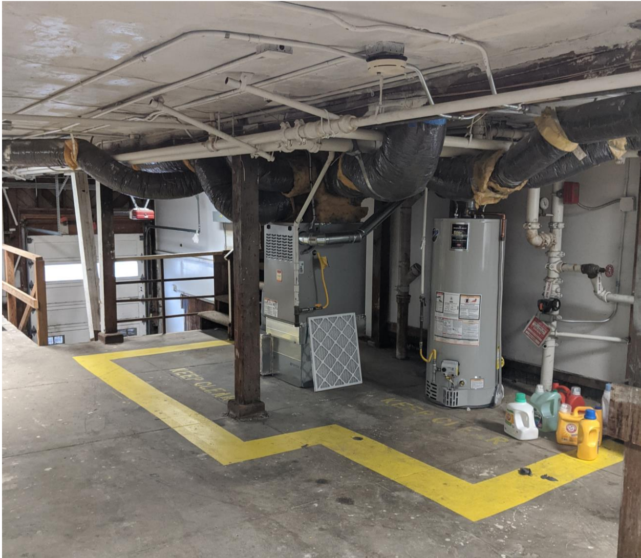
Figure 11 – Unanchored Furnace and Water Heater, both with Flexible Gas Lines
