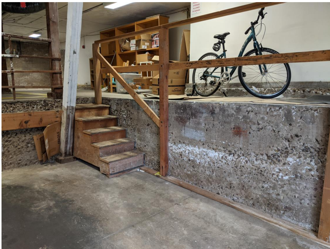
Figure 7 – Concrete Condition at Garage Area
