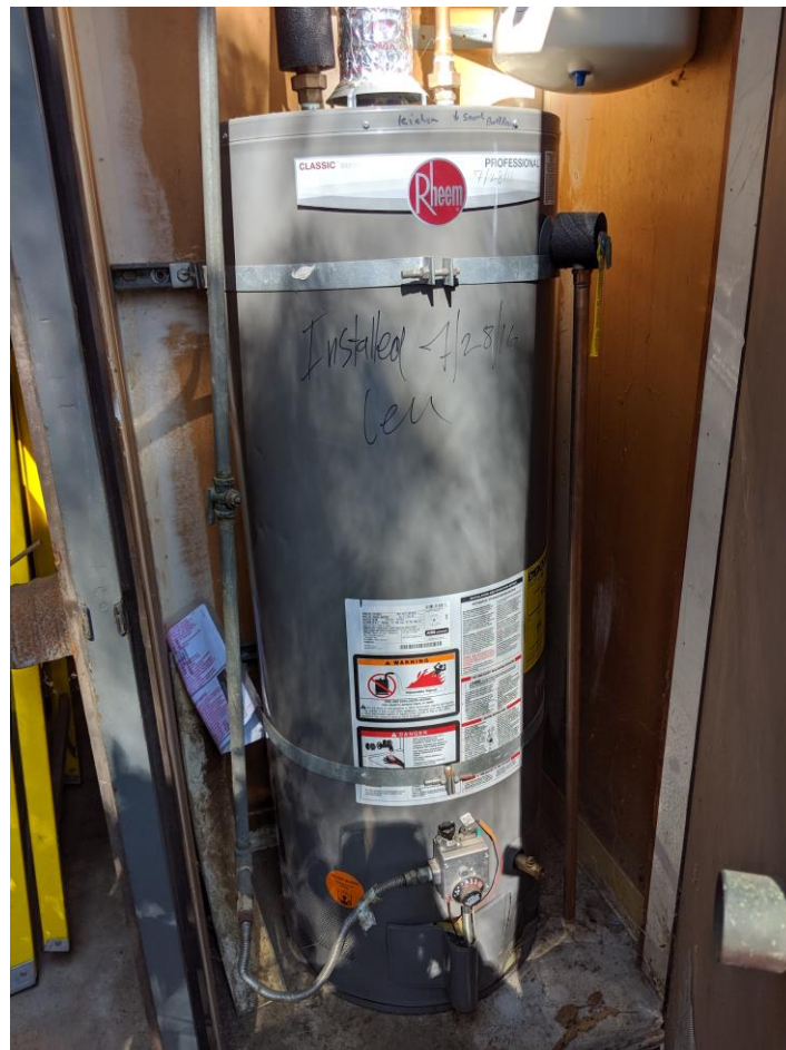
Figure 9 - Braced Water Heater
