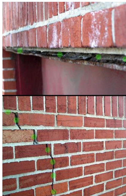
Figure 6. Sections of steel lintel rusting (upper marked by green), and cracking (lower image to the left marked with green) in the brick masonry exterior from Wiss Janney Elstner report on the façade in 2013 showing conditions probably caused by water infiltration at windows.
