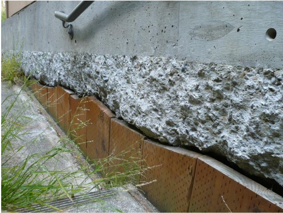
Existing chipped and sloped grade beams on west elevation (possibly to install the stairs in the narrow space available). Beams span to piers.
