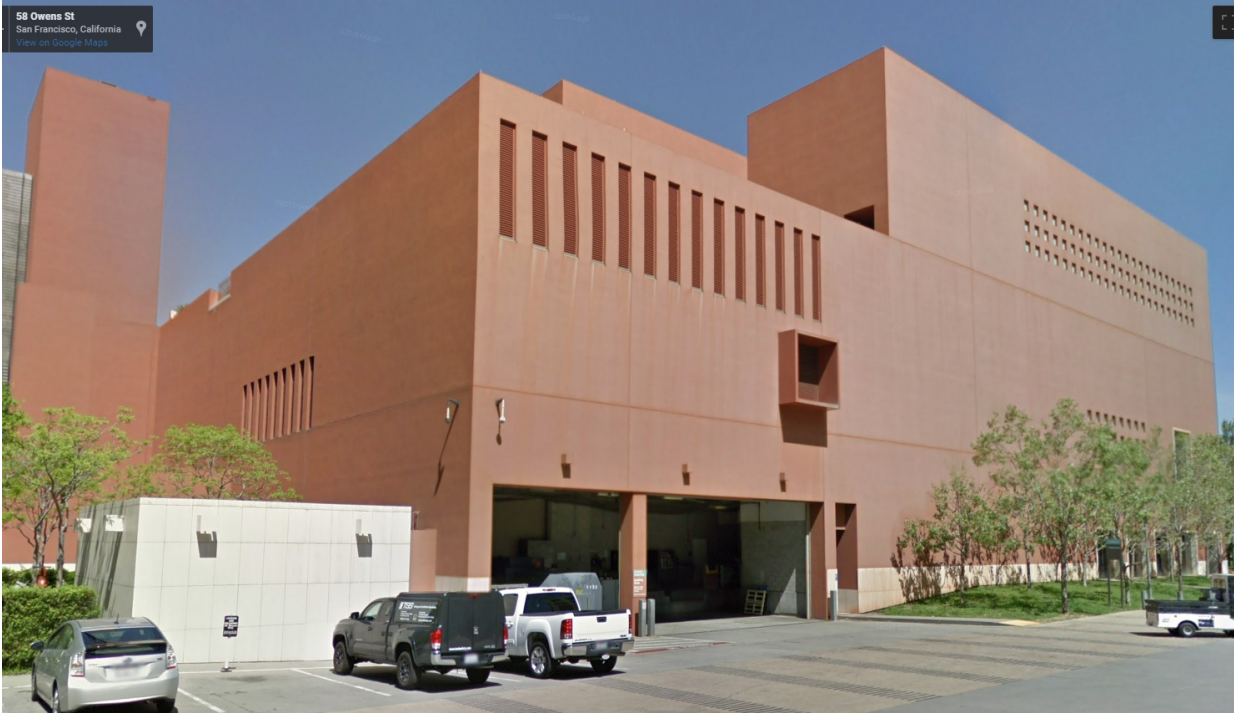
South Elevation (Google StreetView, looking northeast. Transfer girder supports load above loading dock. Stair tower for parking at far left.)
