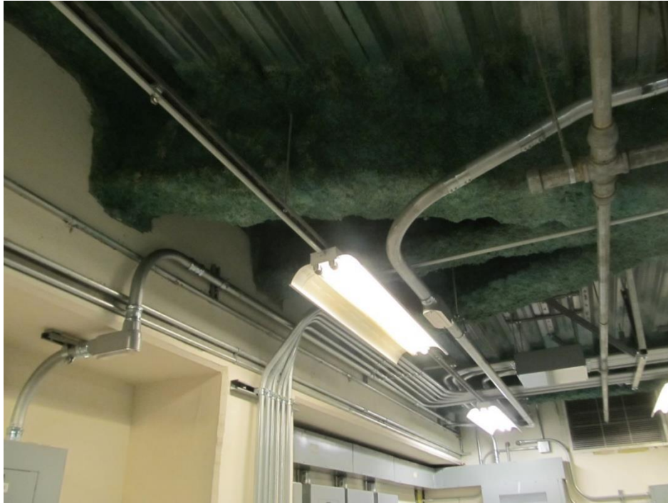
Diagonal steel framing encased in fireproofing provided for lateral bracing of the moment frame beam on the underside of the first floor (looking north)
