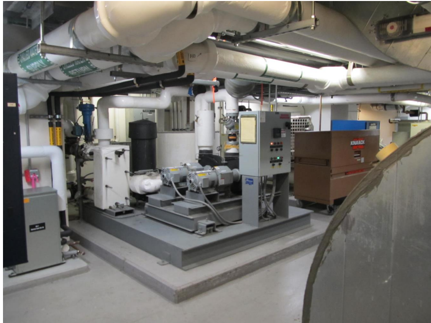
Mechanical room at the mezzanine floor (looking northeast)
