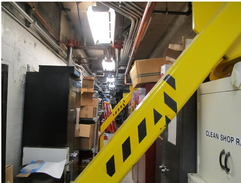
Steel bracing at the mezzanine level Building 'B' on the left and Cancer Center on the right (looking south)
