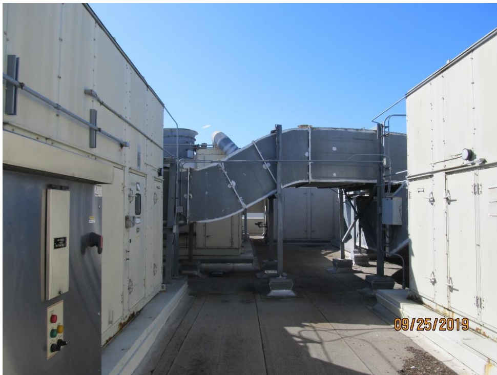
Equipment at the roof (looking south)
