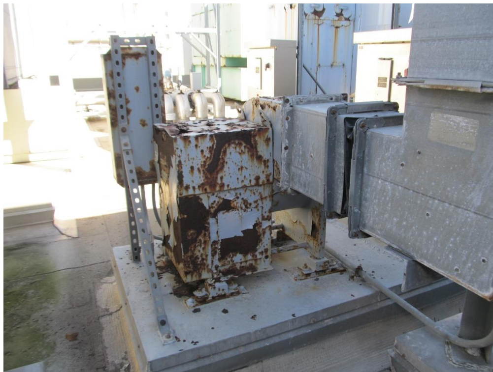
Corroding mechanical equipment at the roof
