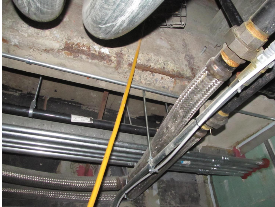
Concrete spalling in void space between Building 'B' and the Cancer Center
