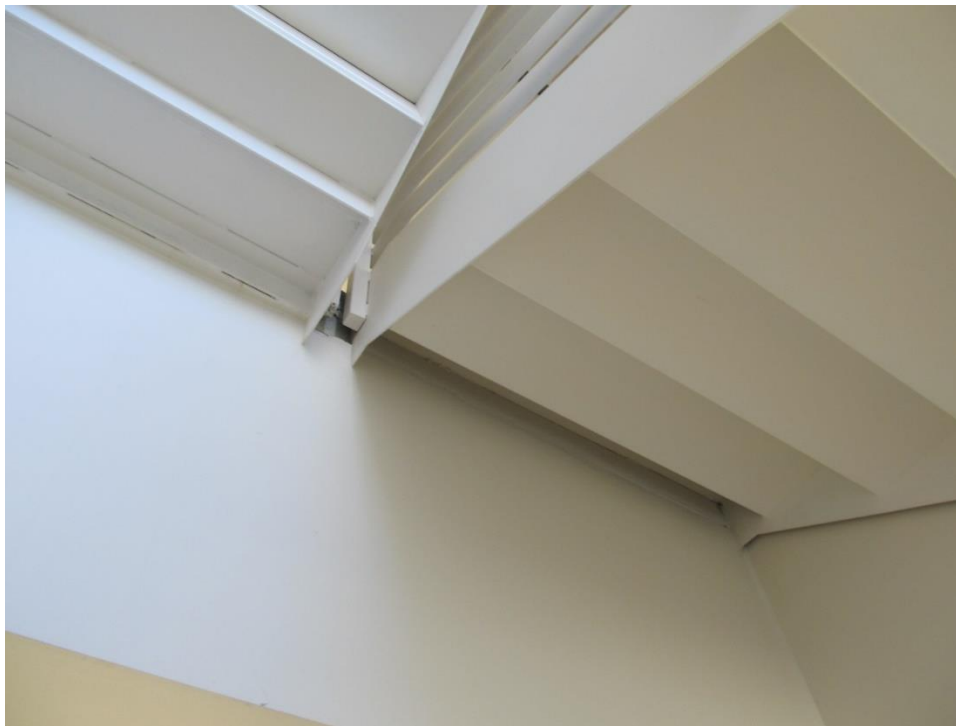
Underside of steel plate stair stringers at the intermediate landing. No slip joint was observed at the floor level or intermediate landing.
