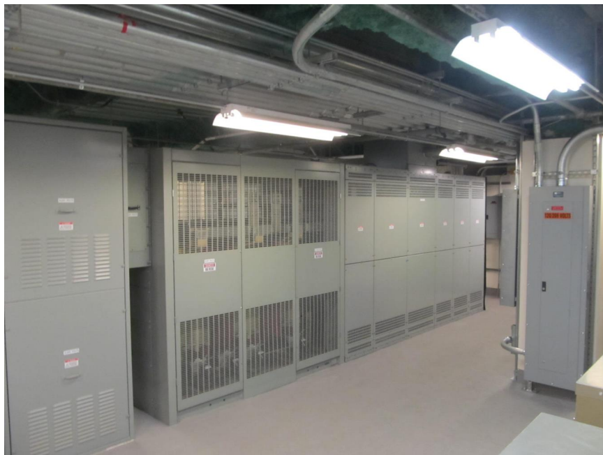
Electrical room at the mezzanine floor (looking northwest)
