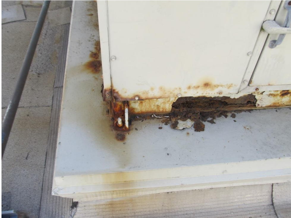
Extensive corrosion at the base of the roof equipment
