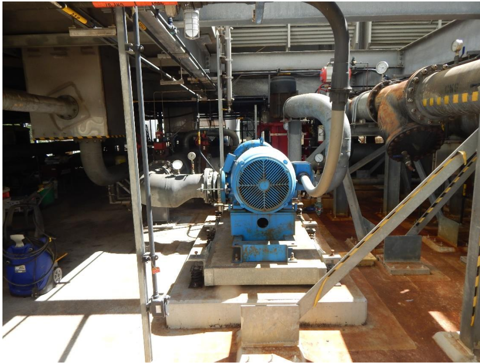
Photo 19. Cooling Tower Pump Anchorage
