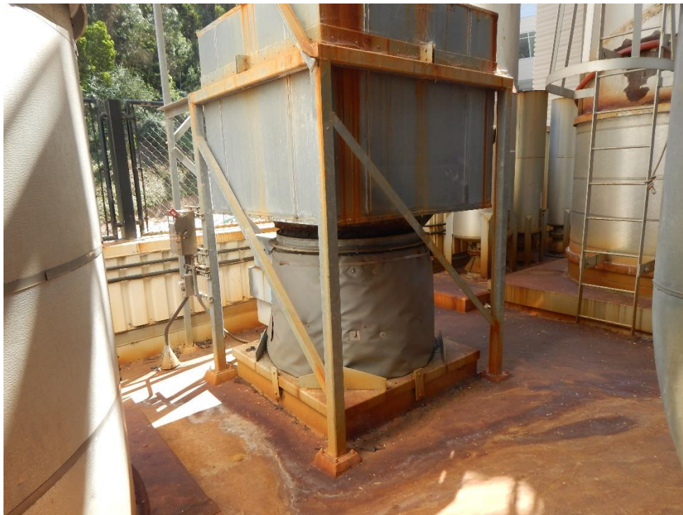
Photo 22. Exhaust Duct Frame
