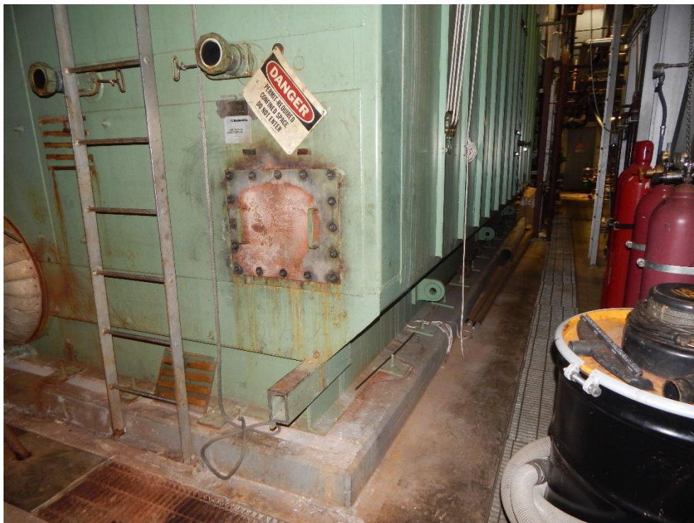
Photo 4. Auxiliary Generator Anchorage
