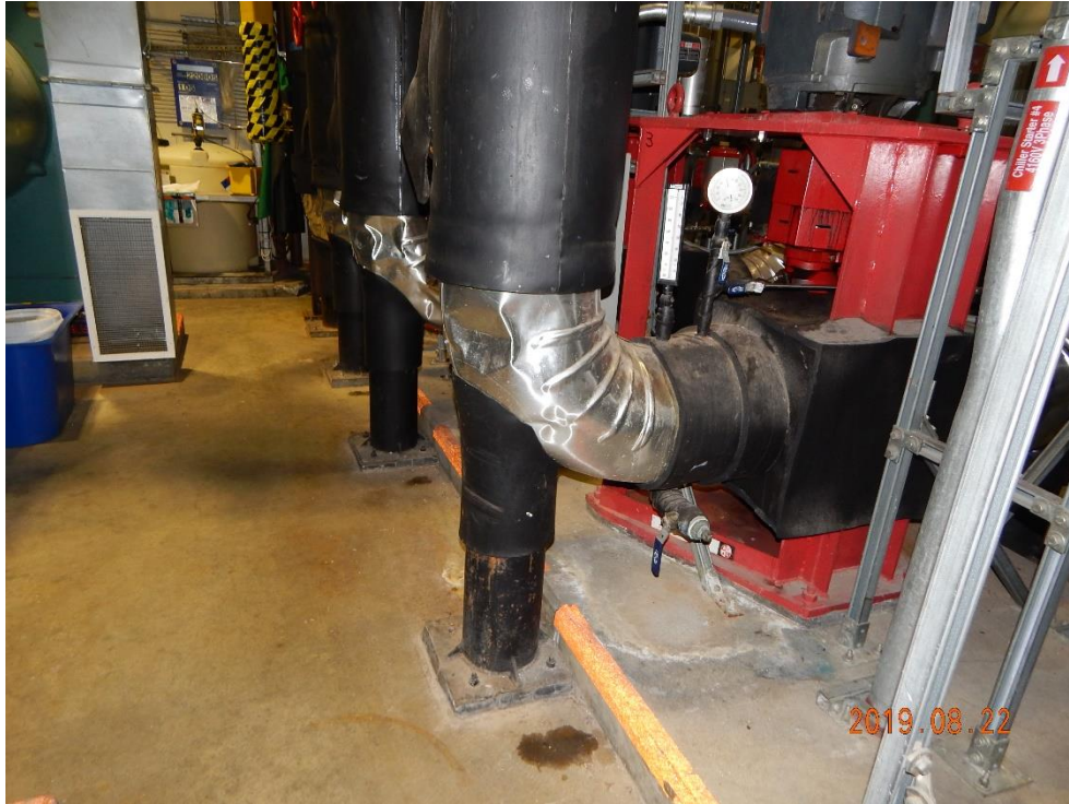
Photo 15. Pump & Pipe Stanchion Anchorage
