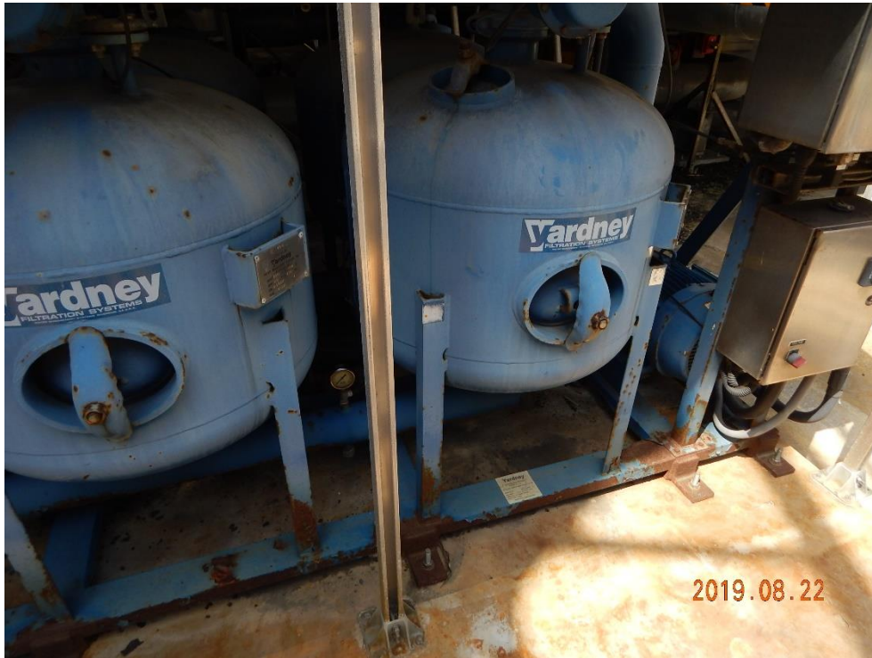
Photo 21. Filtration Tank Anchorage
