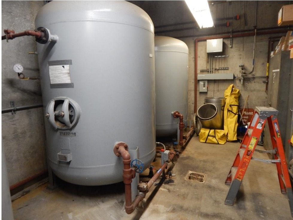
Photo 13. Boiler Tank Anchorage
