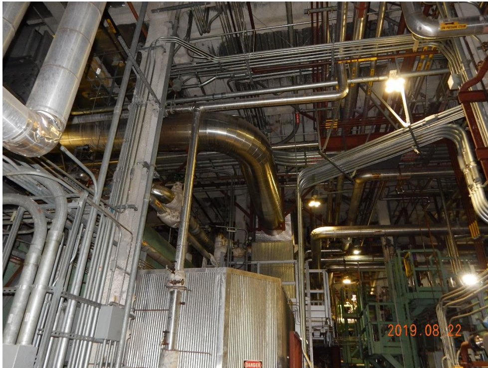
Photo 5. Overhead Pipe/Conduit Bracing
