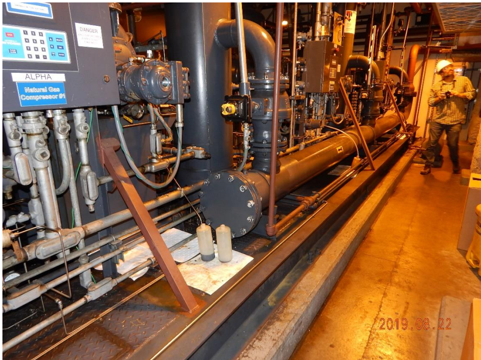
Photo 8. Gas Compressor Skid
