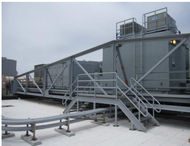
Figure 26: HSE roof equipment bridge and equipment.
