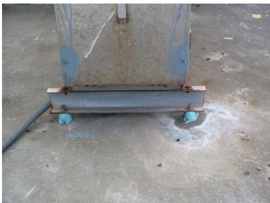
Figure 86: Typical fume exhaust fan HSE with un-restrained rubber isolators.
