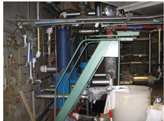
Figure 91: HSW 2nd Floor plumbing room – industrial hot water generator.
