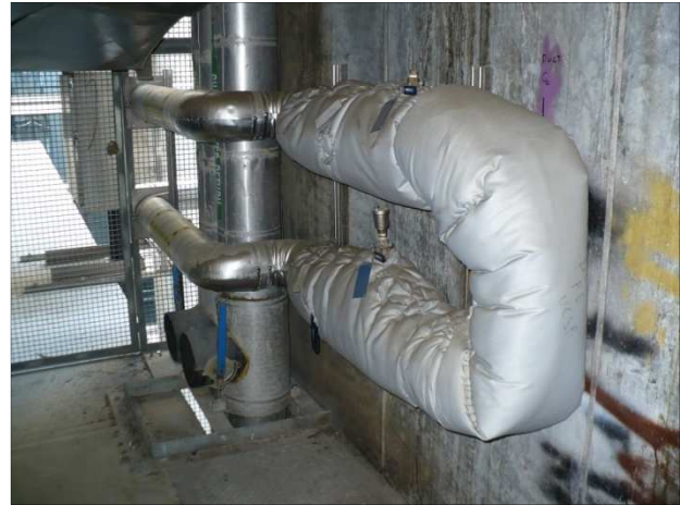
Figure 89: Typical floor chilled water risers through seismic gap with valve stub-outs and heating hot water sub-outs in building gap between stair tower and HSE or HSW.
