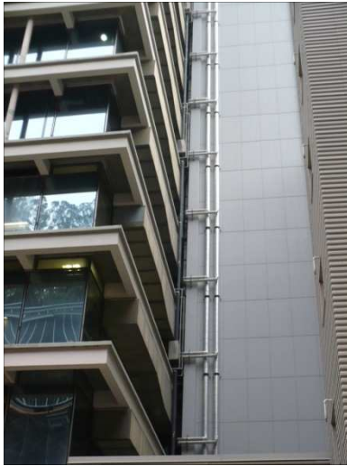
Figure 88: New HSE HHSW/R risers (2000) – south face of stair tower.
