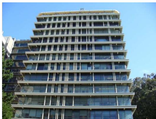
Figure 83: Typical exterior fume exhaust duct risers – HSW north face.
