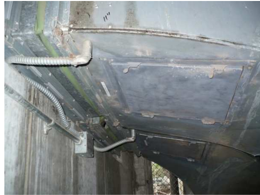
Figure 81: Typical duct penetrations through stair tower shaft.
