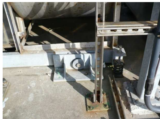
Figure 87: Typical manifolded fume exhaust fan base frame with spring vibration isolators and snubbers.
