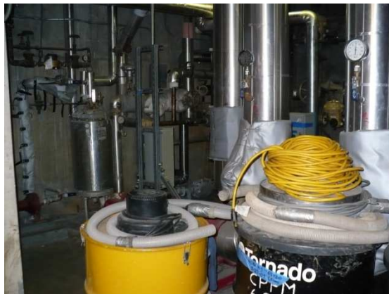
Figure 90: HSE 1st Floor Mechanical Room – domestic hot water generator.
