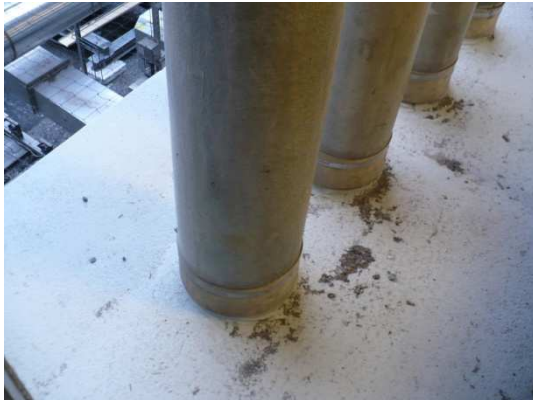
Figure 84: Typical multiple fume exhaust duct risers through the ledge.
