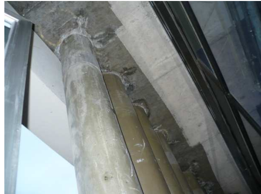
Figure 85: Typical multiple fume exhaust duct risers through the ledge above.
