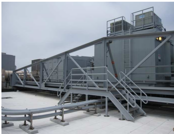
Figure 26: HSE roof equipment bridge and equipment.
