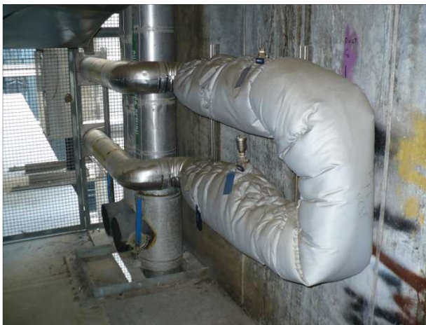
Figure 89: Typical floor chilled water risers through seismic gap with valve stub-outs and heating hot water sub-outs in building gap between stair tower and HSE or HSW.
