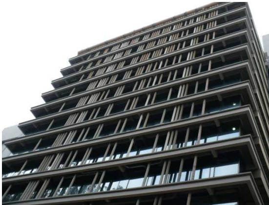
Figure 82: Typical exterior fume exhaust duct risers - HSE south face.
