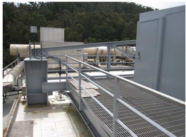
Figure 27: HSE roof equipment bridge column support.
