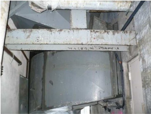
Figure 80: Typical floor main ductwork crossing the separation joint between the stair tower and HSE or HSW.
