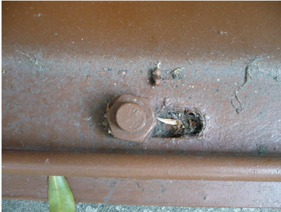
Bridge connection bolt at end of slotted hole. Seismic joint is to the right (west).
