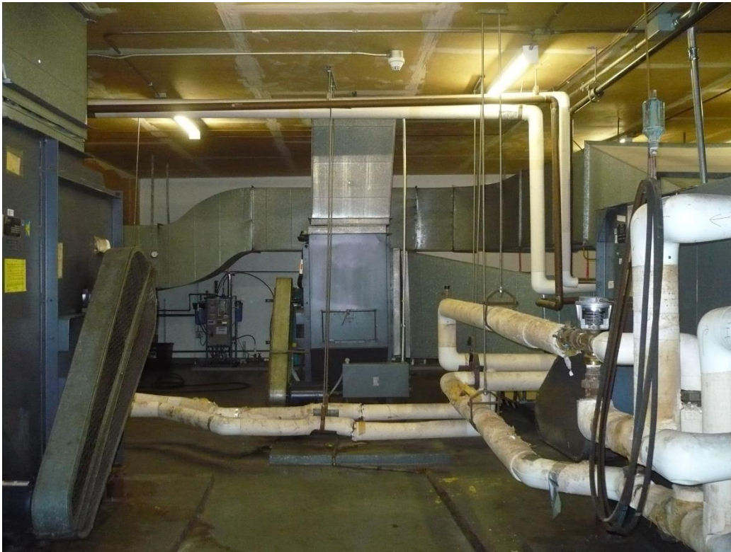
Mechanical room (looking west)
